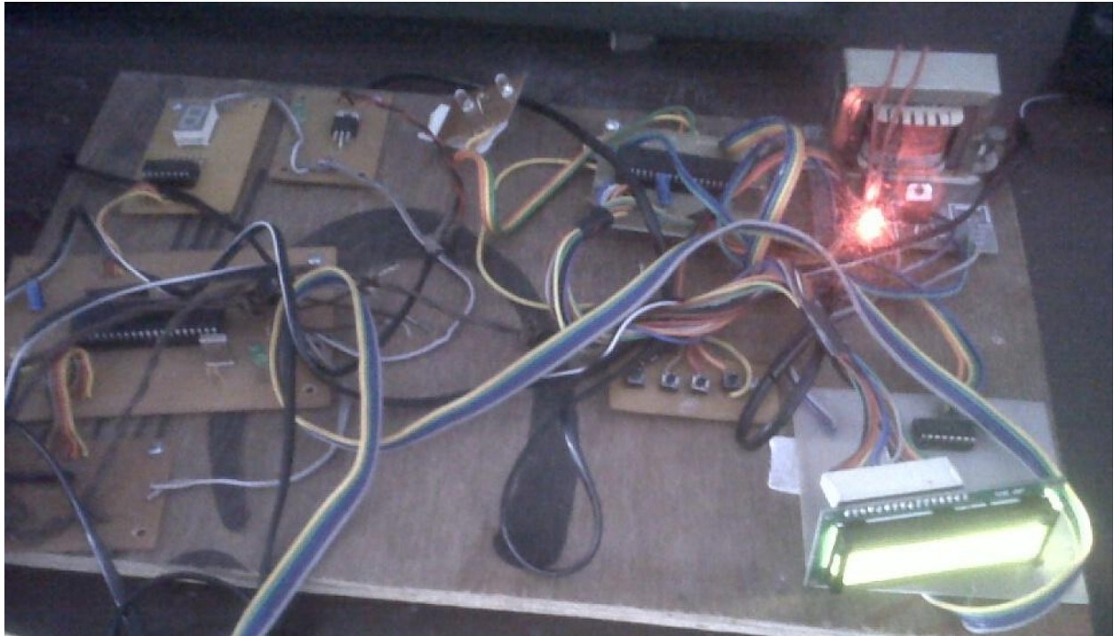
FIGURE 3.13 CONTROL PANEL FOT THE ELEVATOR
