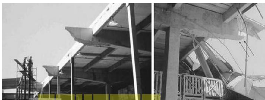
Plate 1.1: Failure of Beams in Shear at Wilkins Air Force Depot, Ohio ( Anderson, 1957 )
