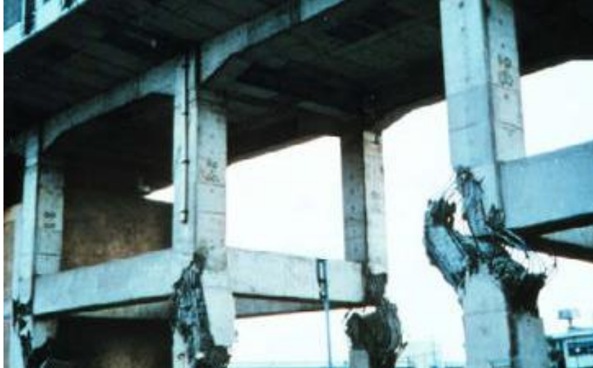
Plate 1.2: Failure of Viaduct Rigid Frame Structure during the Hanshin Earthquake (JSCE, 1995)
