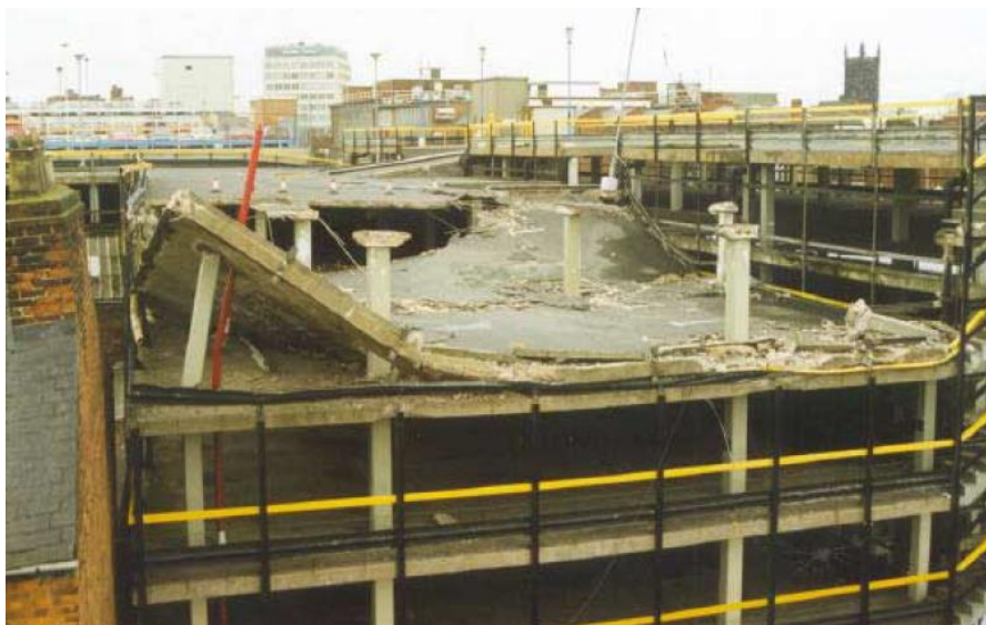
Plate 1.3: Floor Slab Collapsed at Wolverhampton (Wood, 1997)
