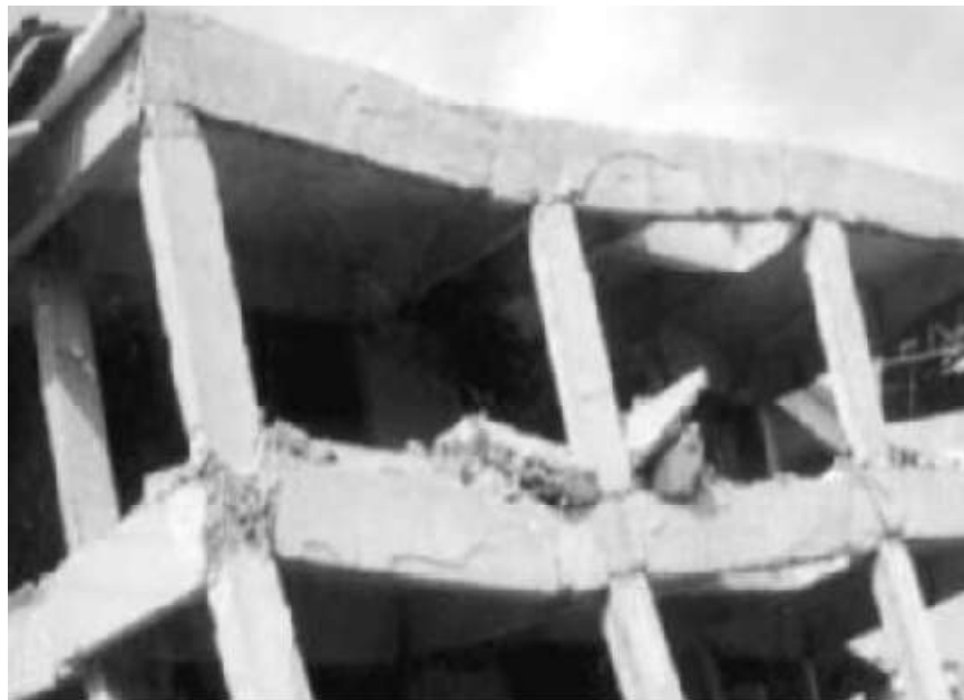
Figure 1.1: Beam-column joint failure due to earthquake (Ghobarah, 2002).
