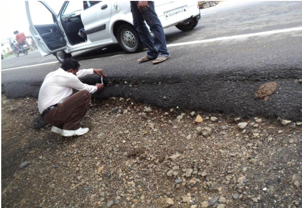
Fig 5. 11 View of Edge Drop at 93+Fig 5.6 View of Edge Drop at 93+300km
