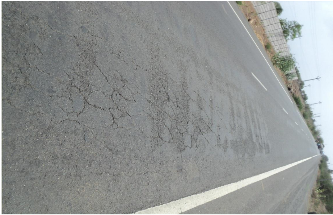
Fig 5. 10 View of cracks with medium severity at 9+300 km.
