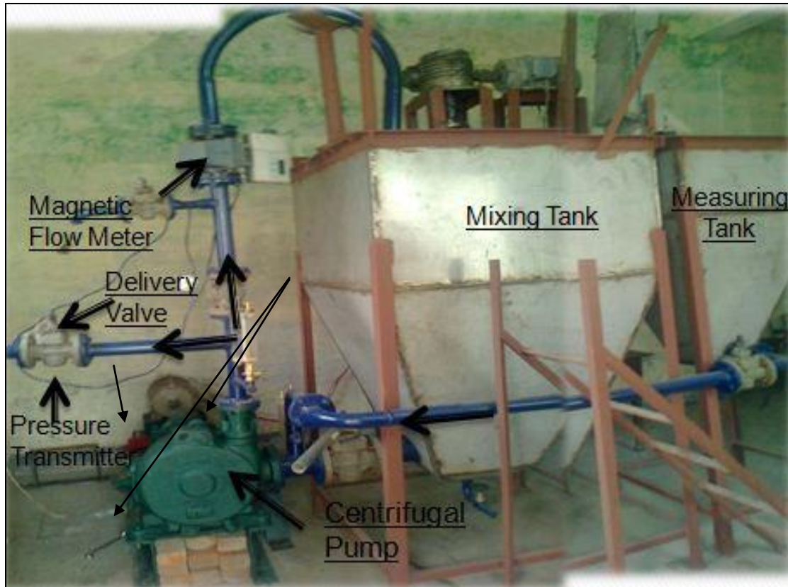
Figure 3.2 Photo graphic view of Centrifugal slurry pump set-up
