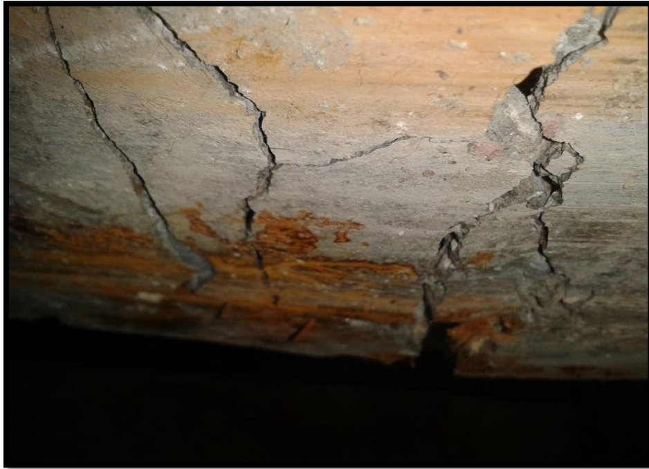
Fig: 5.22 C-12 Beam showing Cracks generated at the soffit after failure
