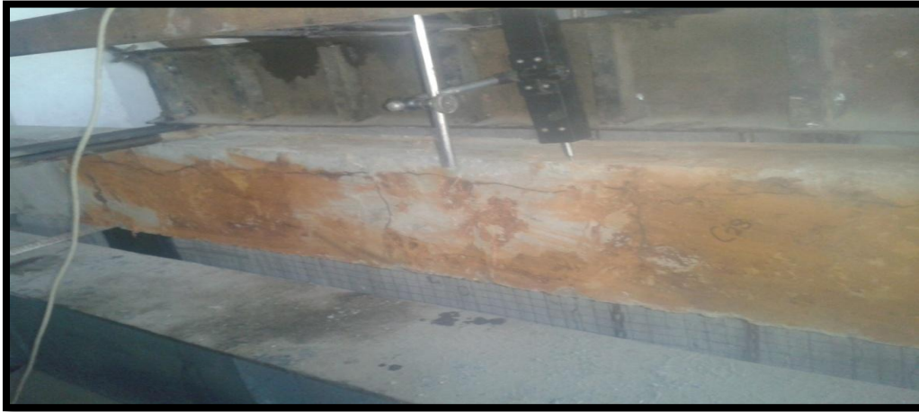
Fig: 5.27 Side face of C-28 Beam before loading
