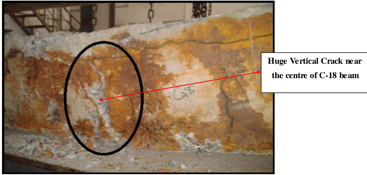
Fig: 5.25 C-18 beam showing large vertical crack near the centre of beam
