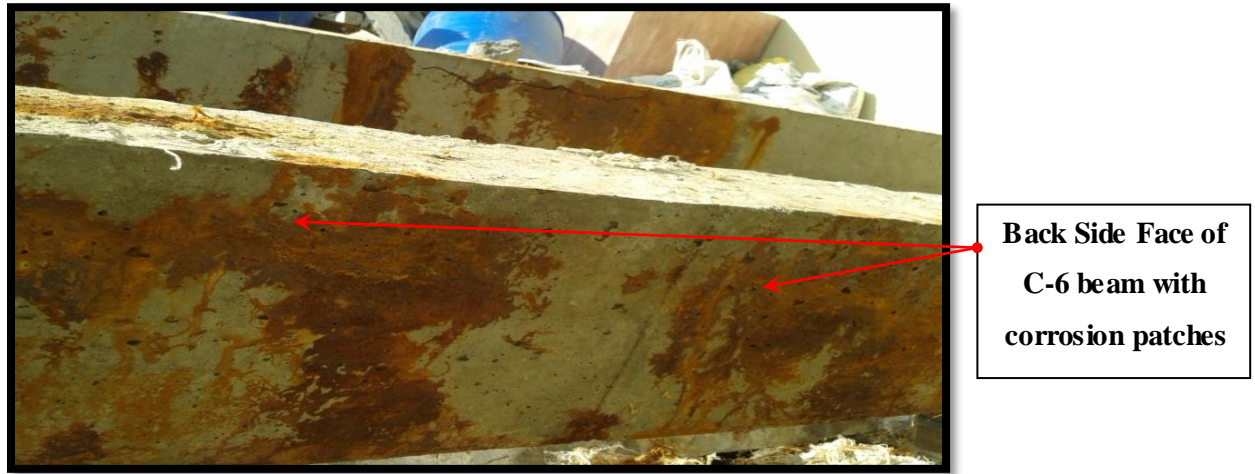
Fig: 5.7 back Side face C-6 beam
