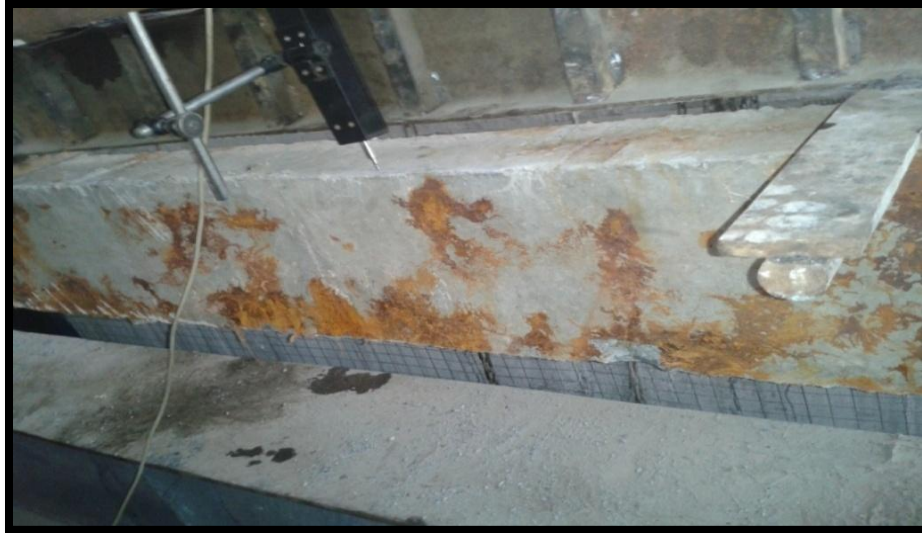
Fig: 5.17 Side face of C-6 Beam before loading
