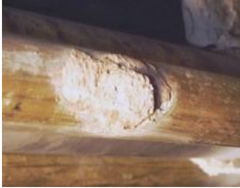
Fig.1.13: Stray Current Corrosion [4]
