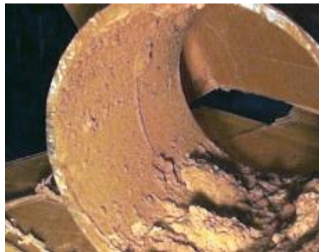
Fig. 1.16: Thermo galvanic Corrosion [4]
