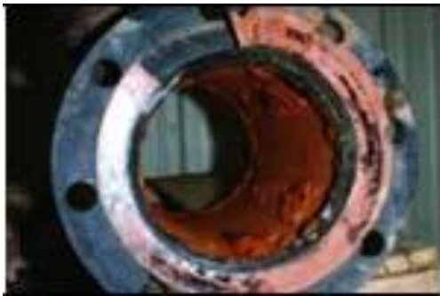
Fig .1.14: Microbial Corrosion [4]
