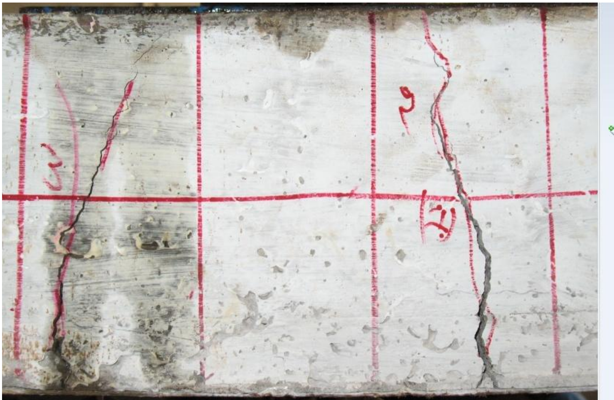
Fig.7.35 Widening of cracks at 200kN
