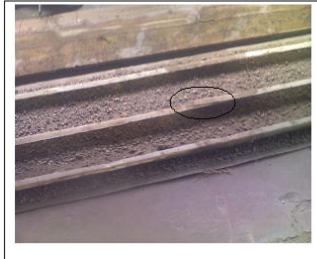
Fig 7.23 Delamination of the second connector layer
