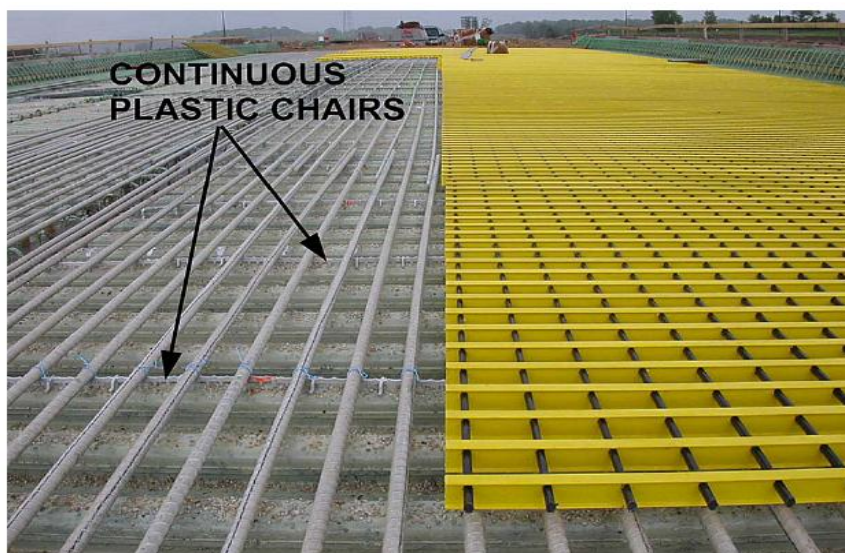
Fig.3.23. SIP FRP deck panels, FRP rebars, and bi-directional FRP grid during placement (Berg et al., 2005)
