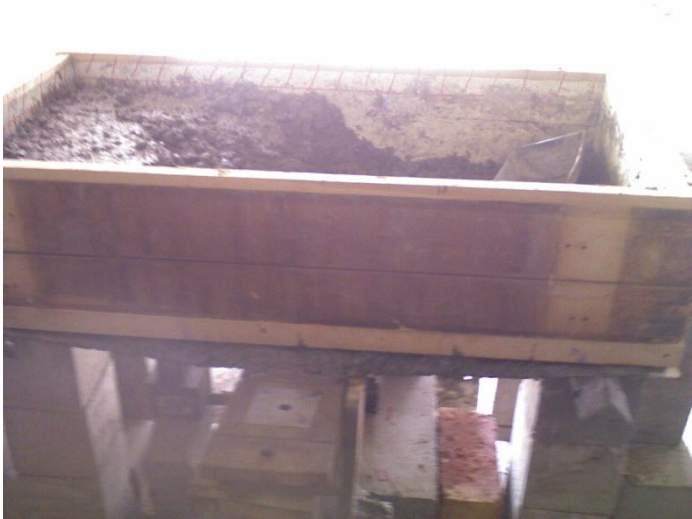
Fig7.8. Excessive deflection of form D21
