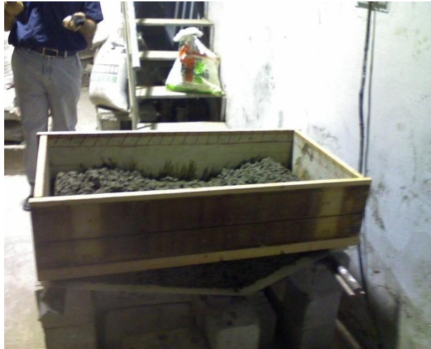
Fig 7.3 Excessive deflection during slab casting on form D11
