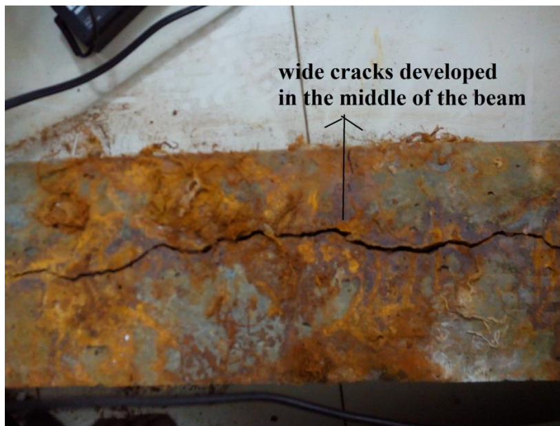
Fig.4.36: Cracks developed in specimen after 30 days of accelerated corrosion.
