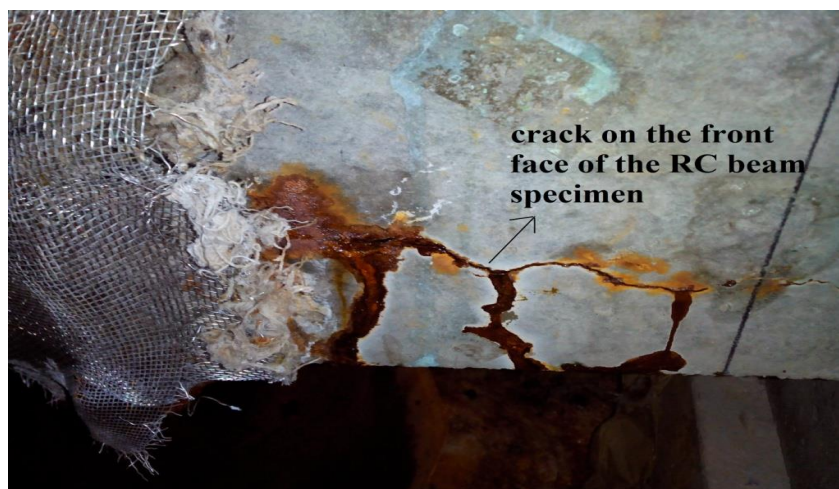
Fig.4.30: Condition of specimen after exposure to 20 days of accelerated corrosion
