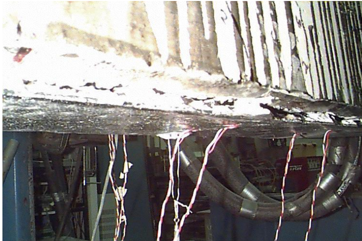
Figure 2.8 Debonding of the CFRP (Carlin, B. P., 1998)
