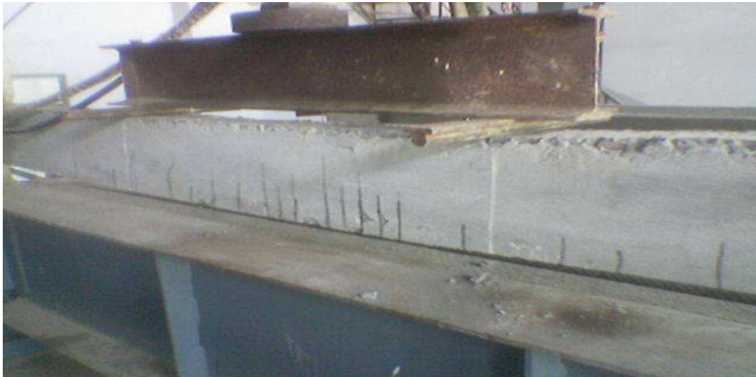
Plate 4.2: Crack Pattern of Retrofitted Beam with 0 Degree Wire Mesh
