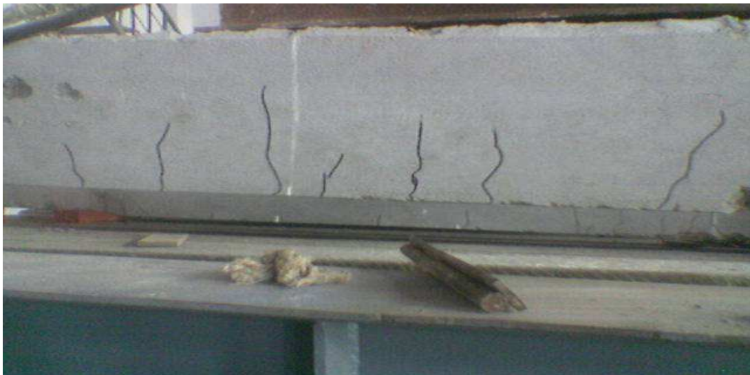
Plate 4.4: Crack Pattern of Retrofitted Beam with 45 Degree Wire Mesh
