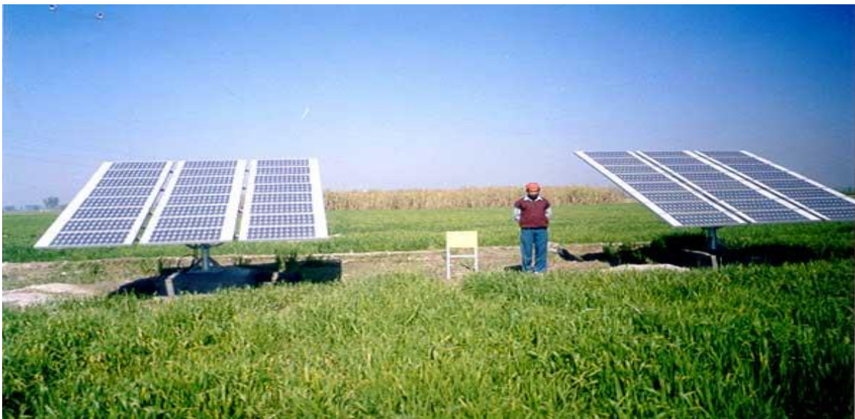
Figure 4.5 A solar pump installed in one of the village
