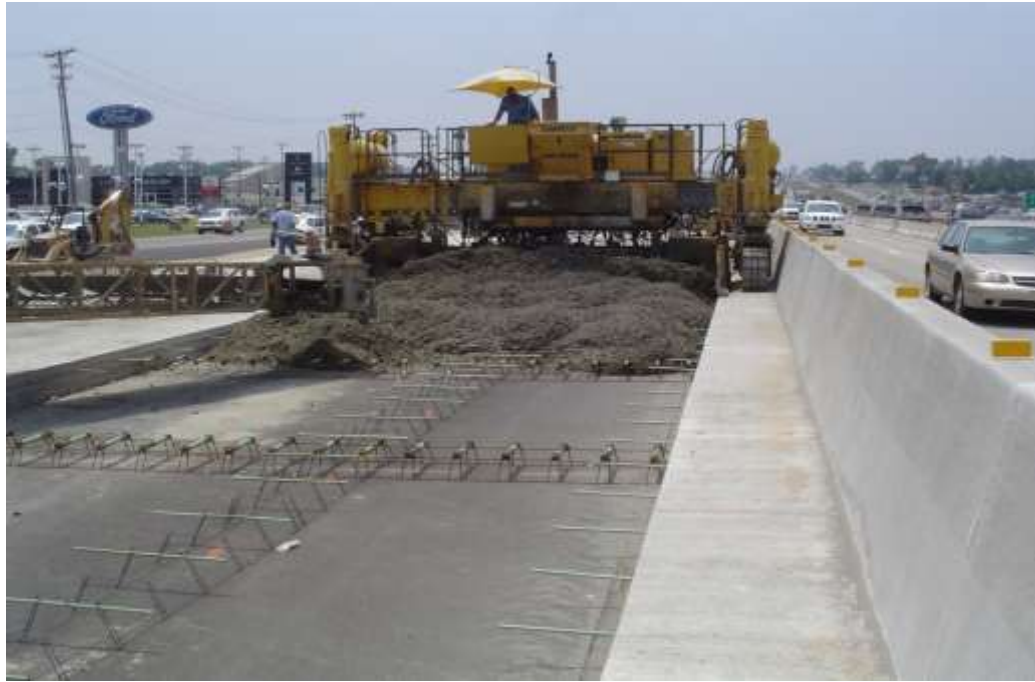
Fig. 1.10 Placing of Dowel bars manually and Laying of Pavement Quality Concrete with paver.
