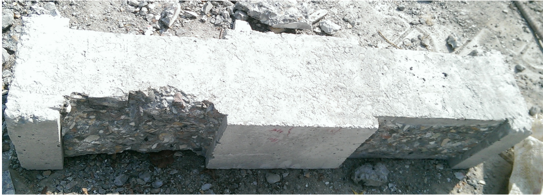
Fig. 3.8 Side Face Chipped off Beam (Stage 1)
