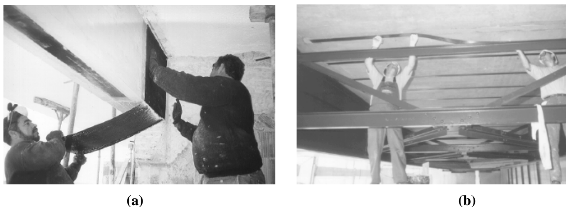
Fig. 1.6: (a) Hand lay-up of CFRP sheets or fabrics; (b) Application of prefabricated strips.
