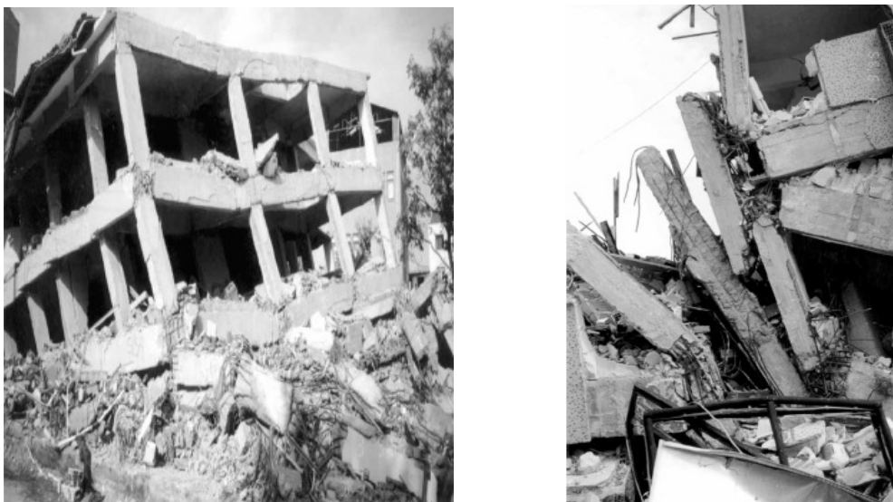
Fig. 1.2: Typical beam-column joint failures (1999 Turkey earthquake).
