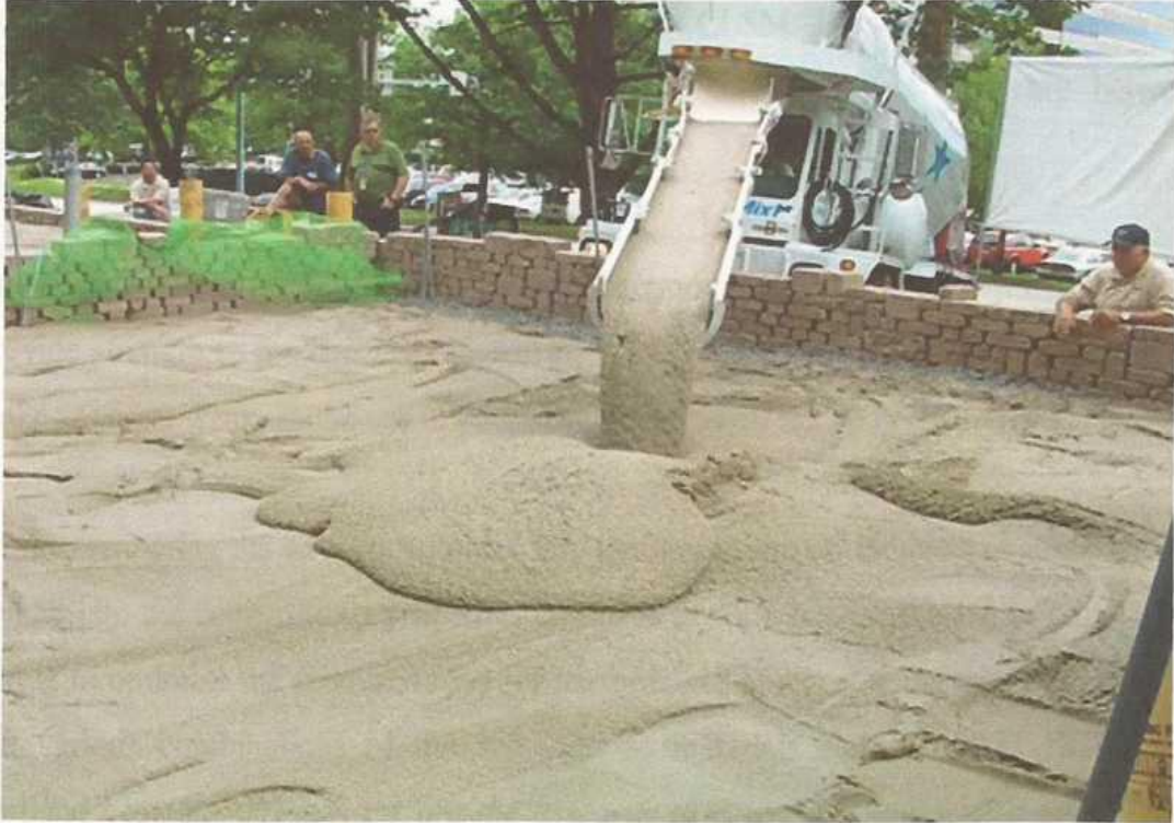
Figure 2.5 - 'Cement/PFA CLSM mix' flowing down the chute of a ready mix truck
