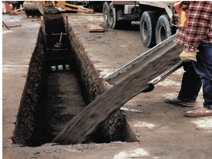
Figure 2.1 - Flowing down the chute of a ready mix truck, CLSM quickly fills this deep utility trench.
