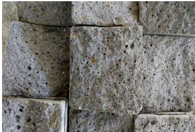
Fig 3. 6:Voids Present in Mortar Sample
