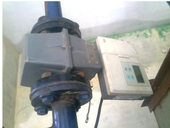
Figure 3.4 Electro-magnetic Flow Meter
