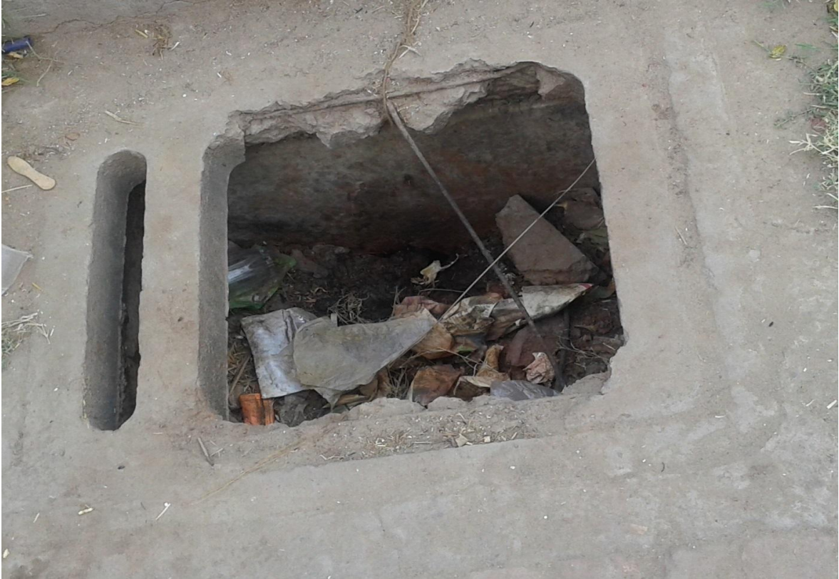
Figure 4.3: Choked Drain near Petrol Pump on Road Section UR-01
