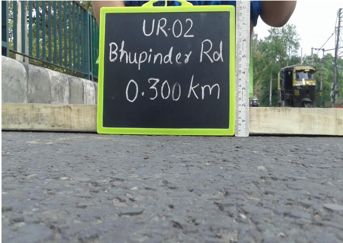
Figure 4.20: Rut Depth Measurement at chainage 0.300 km on Section UR-02
