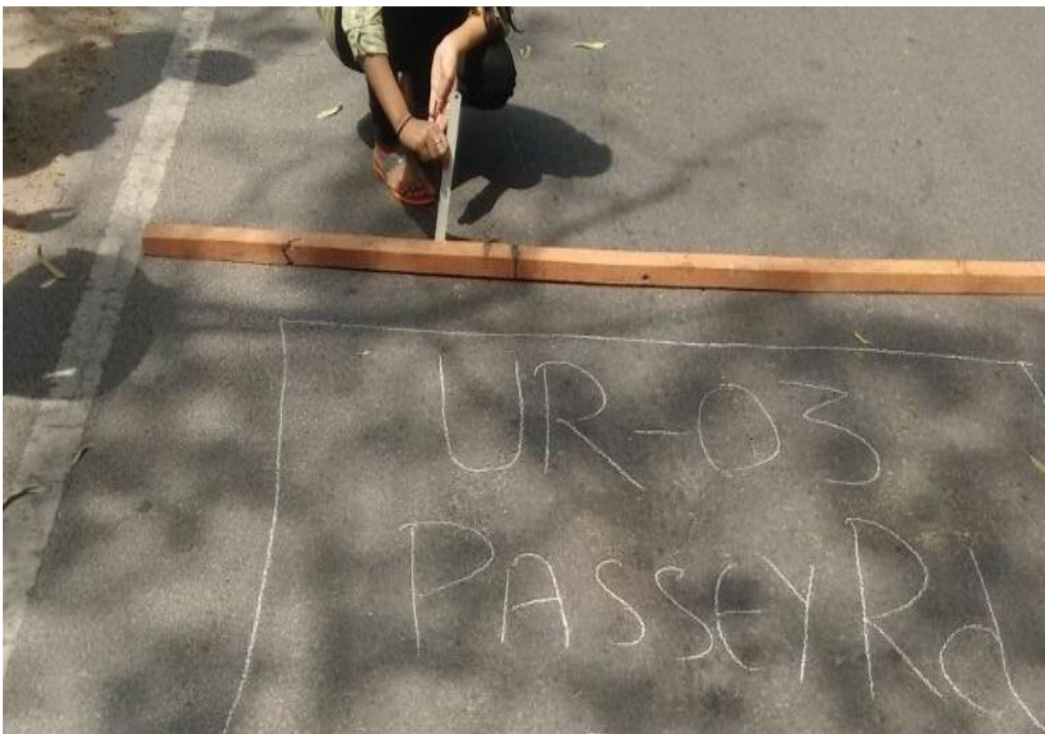
Figure 4.21: Rut Depth Measurement at chainage 0.400 km on Section UR-03
