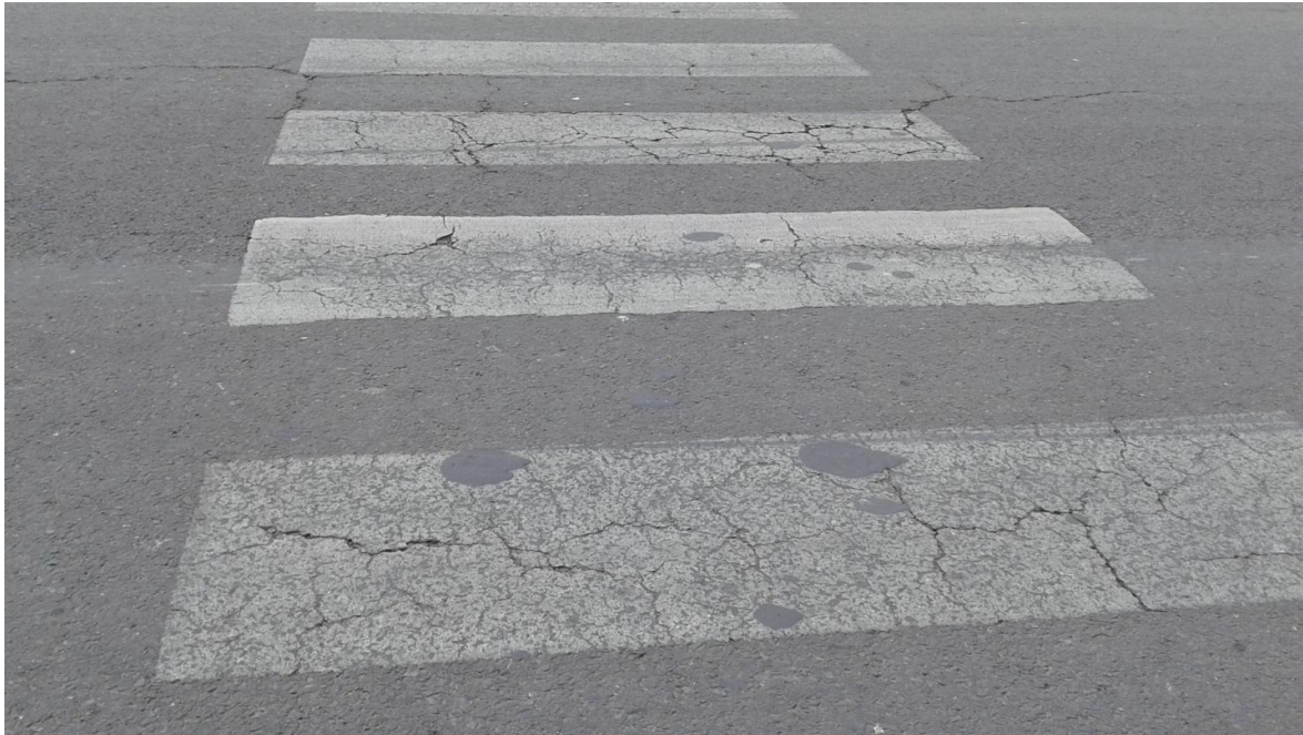
Figure 4.13: Cracks on Road Section UR-03
