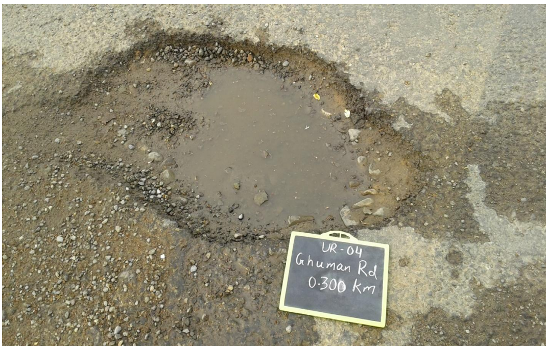
Figure 4.18: Pothole at Chainage 0.300 km on Section UR-04
