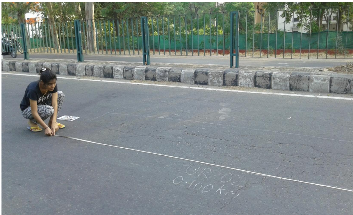
Figure 4.14: Crack Measurement with tape at chainage 0.100 km on Section UR-02
