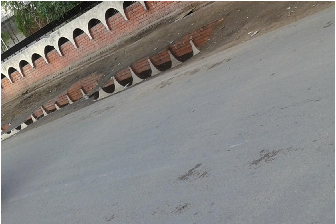
Figure 4.4: Still Water on Shoulder near Kababchi Restaurant on Road Section UR-02
