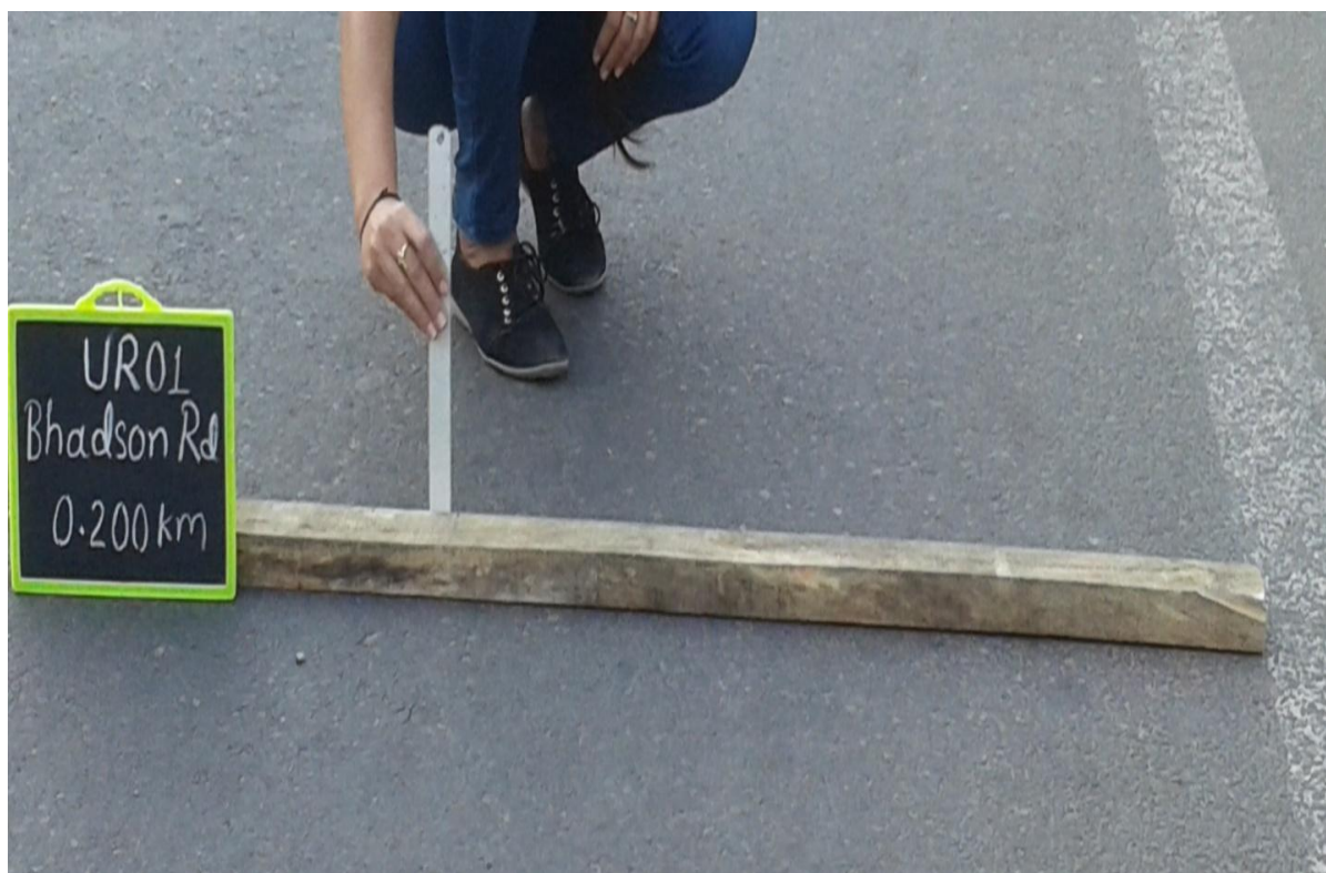
Figure 4.19: Rut Depth Measurement at chainage 0.200 km on Section UR-01
