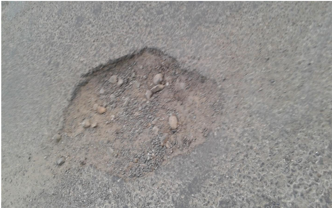
Figure 4.17: Pothole at Chainage 0.850 km on Section UR-02
