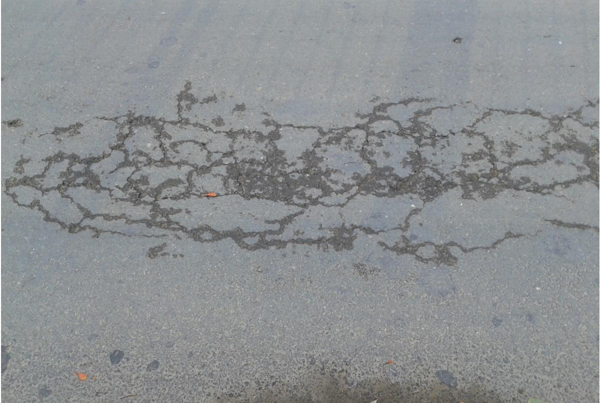
Figure 4.15: Cracks at chainage 0.050 km on Section UR-04
