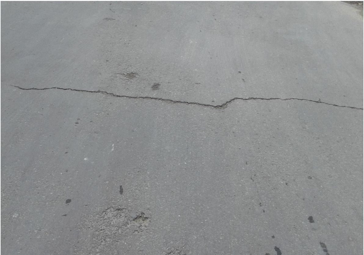
Figure 4.16: Wide Transverse Crack on Section UR-04
