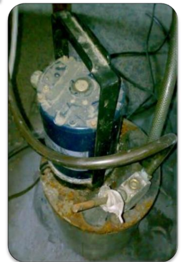
Figure 3.5 Pump for re-circulation of abrasive slurry
