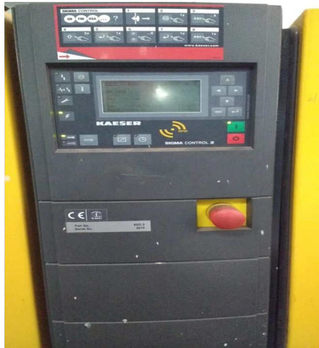
Figure 4.5: picture of VFD
