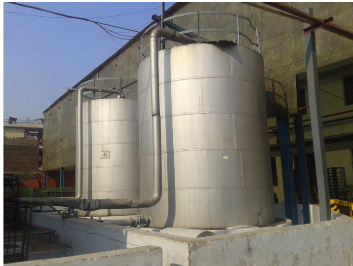
Figure 4.8: picture of storage tank
