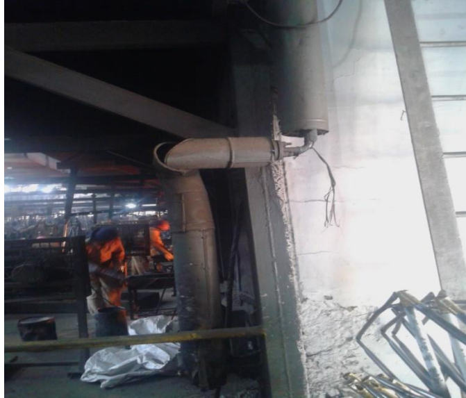
Figure 4.10: picture of electrical heater
