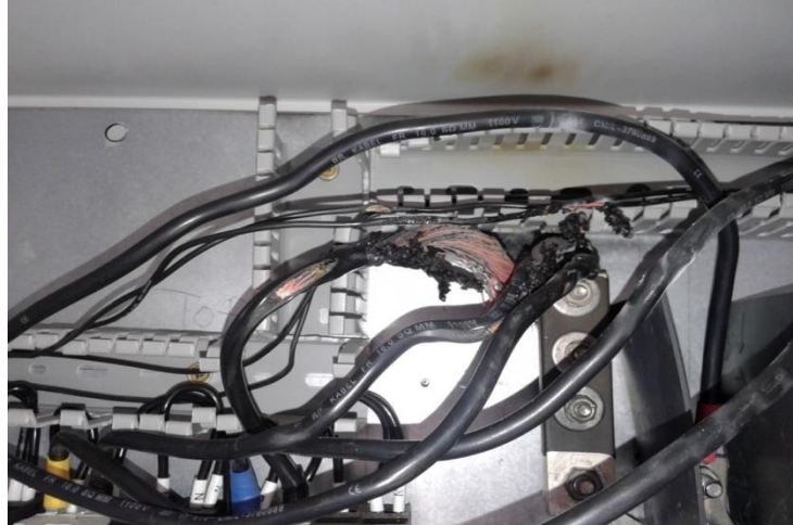
Figure 4.18: faults in grid box
