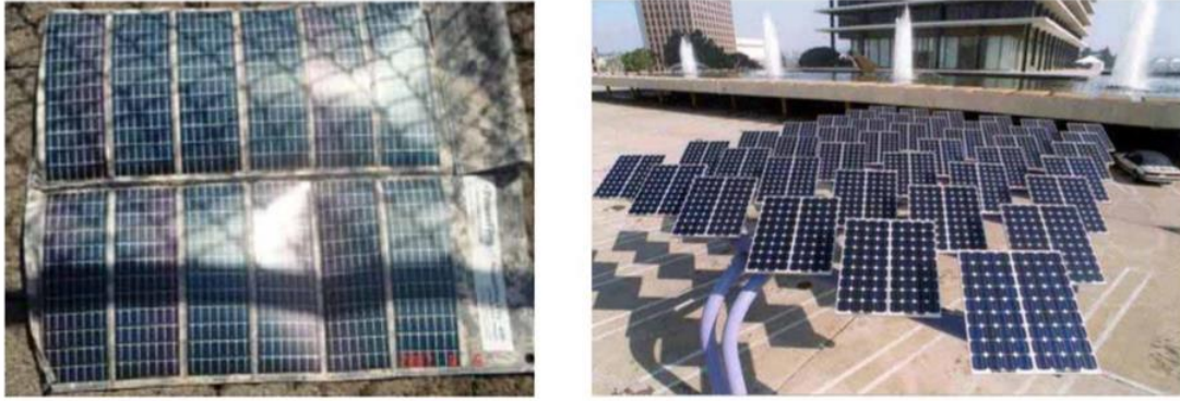
Figure 2.3: Solar panels and modules
