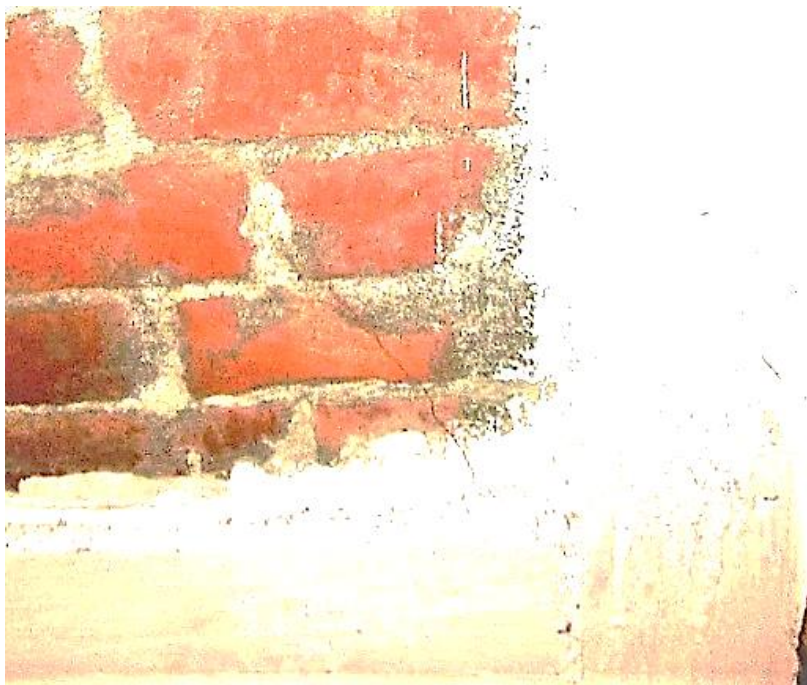
Figure 5. 9: Cracks observed at lower end at 2.1% drift in specimen “B”
