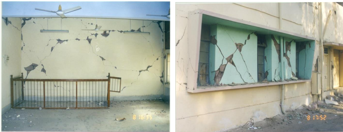
Figure 1. 1: Failure of masonry walls (a) In-plane failure of wall of District court building at Bhuj (Dubey, R.N., 2011); (b) Diagonal cracks in the short pier in Zila Panchayat building at Bhuj (Dubey, R.N., 2011)
