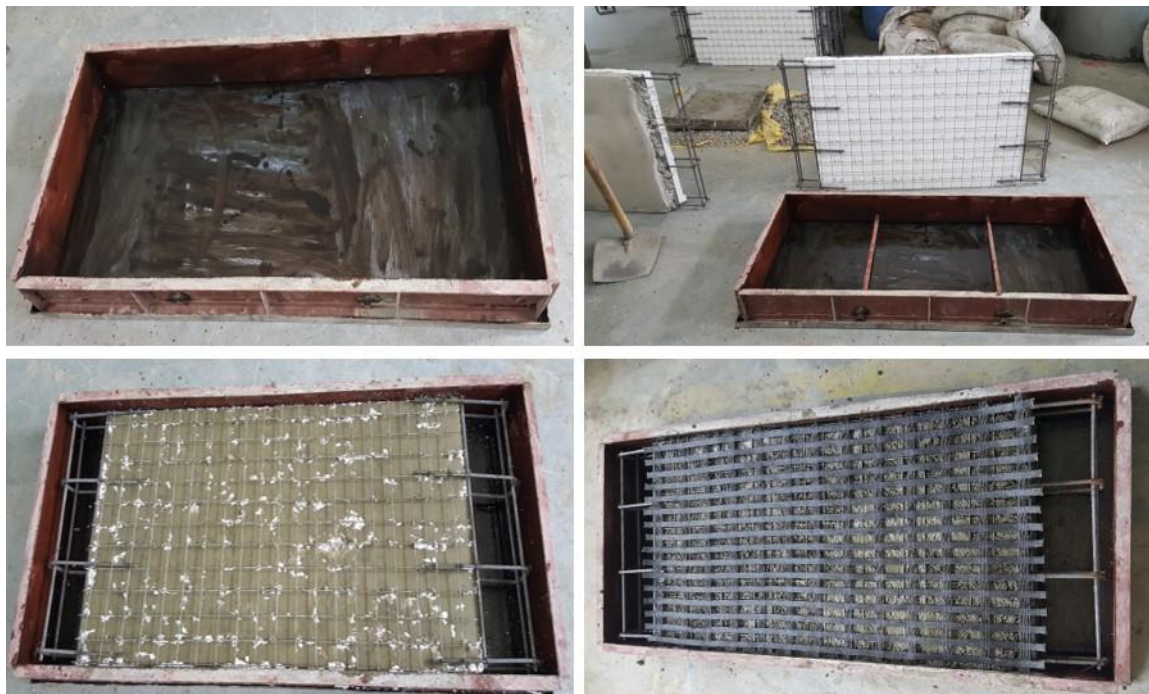
Figure 3. 24: Casting of axial compression specimen (a) Steel mould for casting of specimen; (b) mould with rods to support the panel to help in casting of first layer; (c) rich slurry mix spread over the core of sandwich panel
