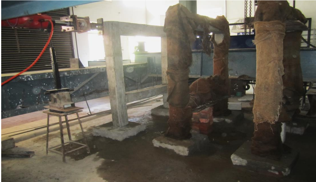
Figure 3. 37: Three bare 2D RC frames under going curing with the help of gunny bags
