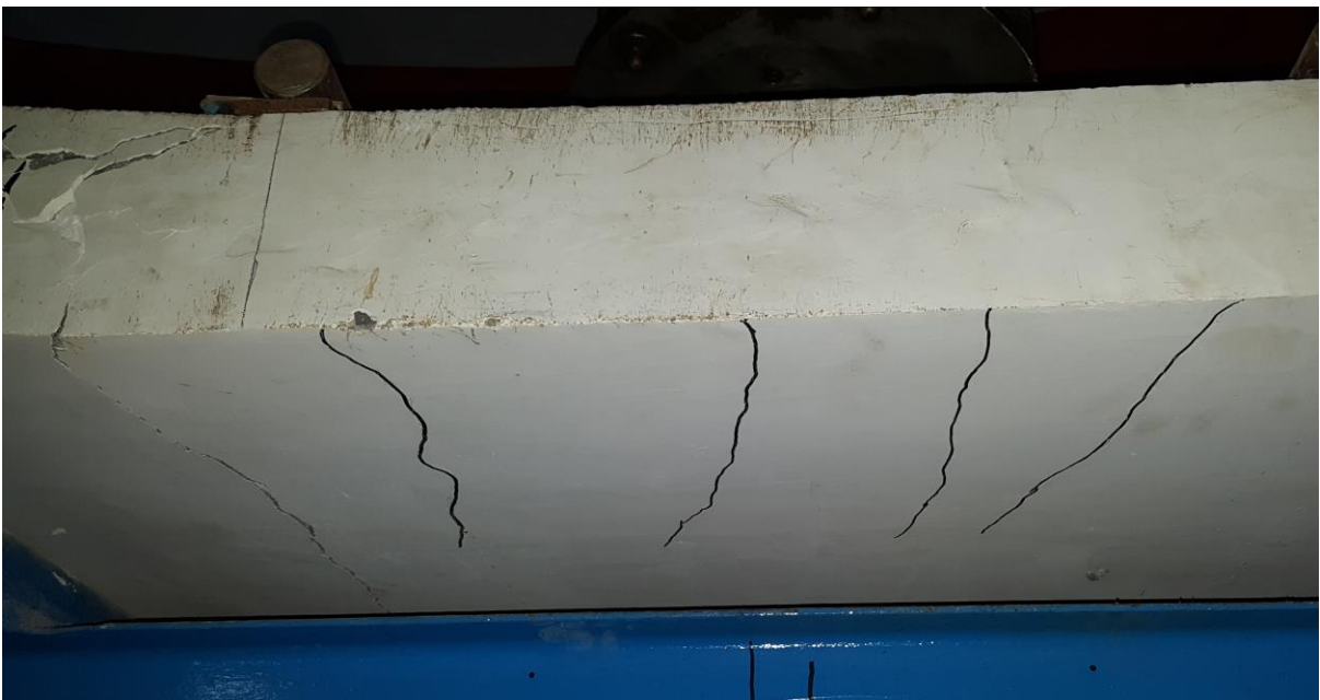
Figure 4. 8: Flexural crack running throughout the width of the specimen in the bottom wythe
