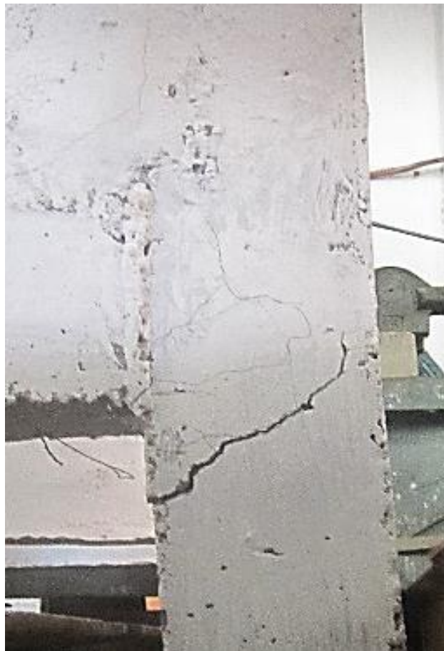
Figure 5. 7: Specimen “C” having a flexural failure in column
