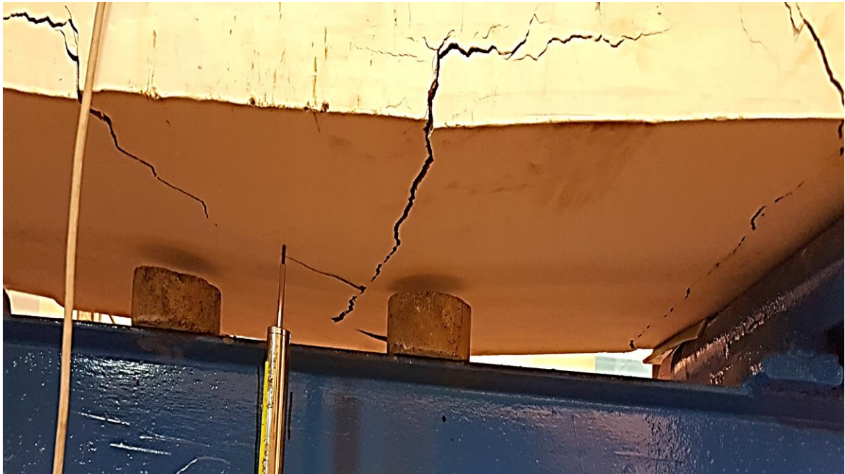
Figure 4. 6: Crack width expansion
