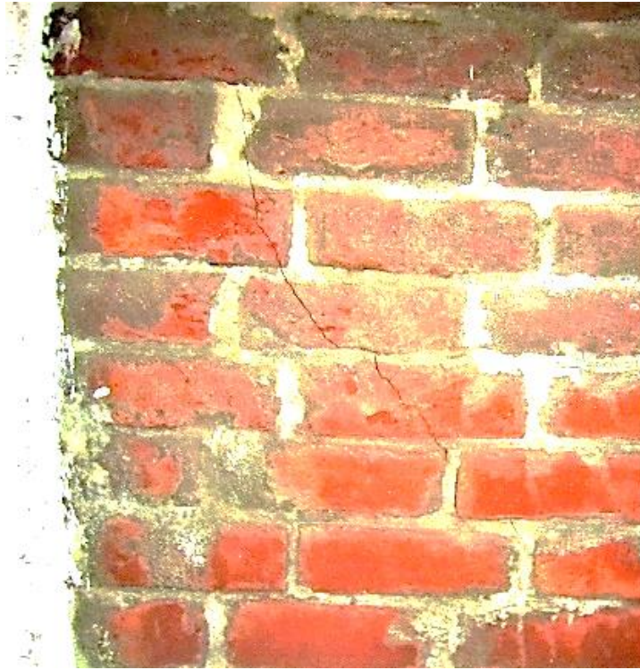
Figure 5. 8: Diagonal cracks propagating from top left corner to middle in specimen “B”
