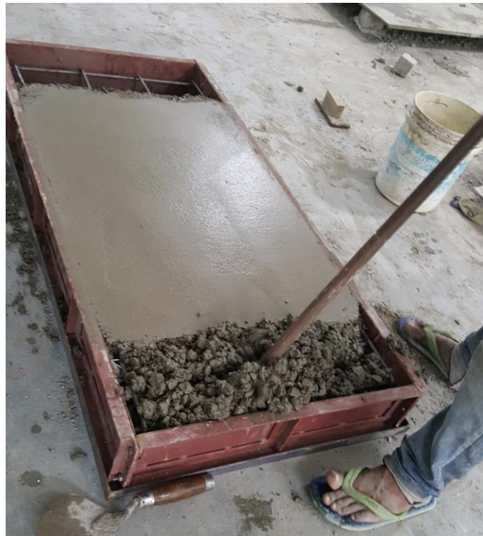
Figure 3. 26: Casting of end beam with M20 mix, a steel rod is being used for compaction of the concrete.
