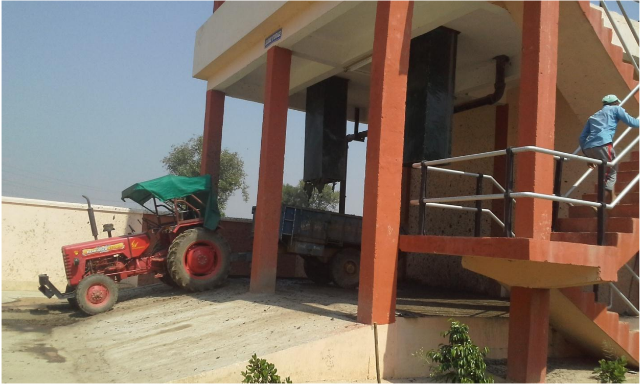
Fig 3.23 Collection Point under Centrifuge Unit (at STP Ablawal)
