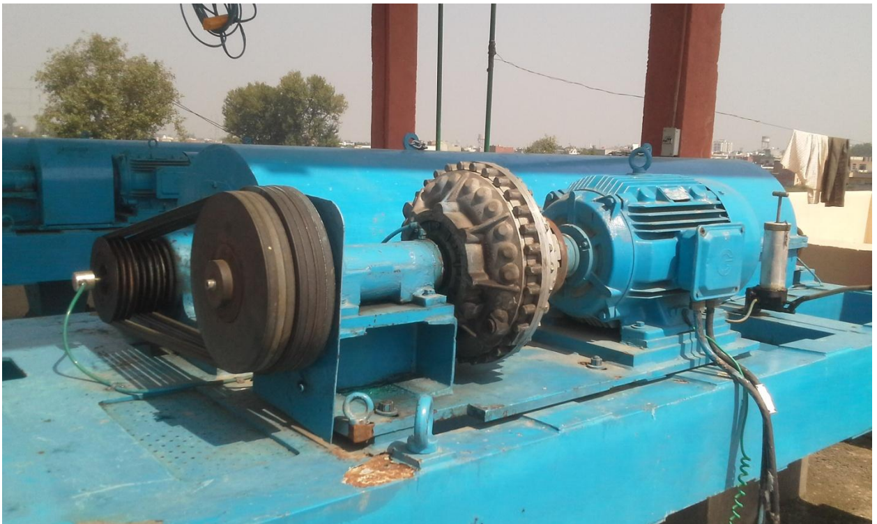
Fig 3.22 Motor Rotating Centrifuge Unit
