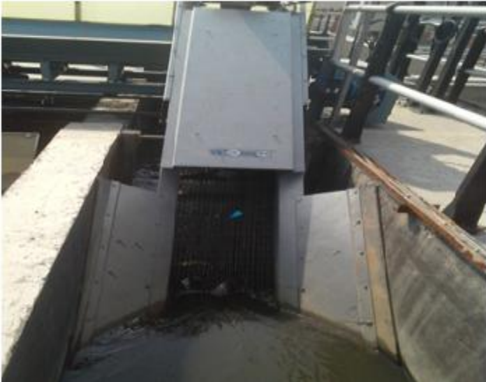
Fig 3.11 : Grit Removal Unit
