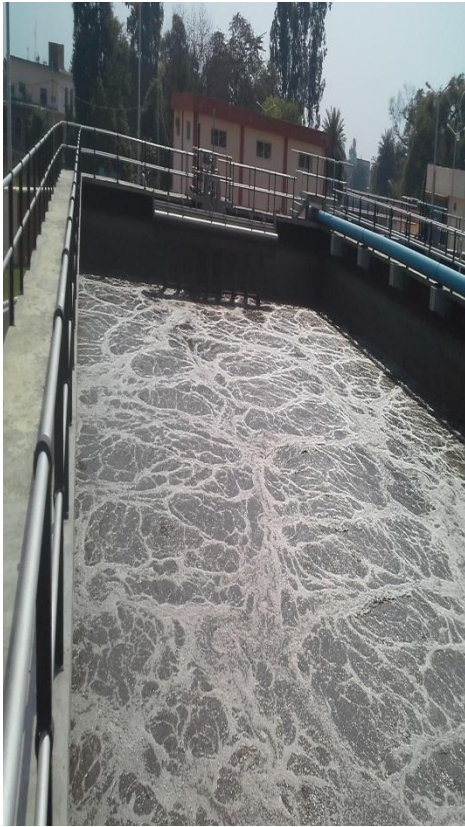
Fig 3.16 Aeration Pond Fig
