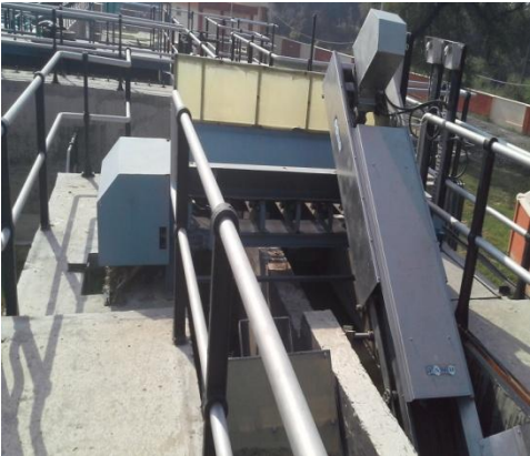
Fig 3.12 Grit Removal Machinery
