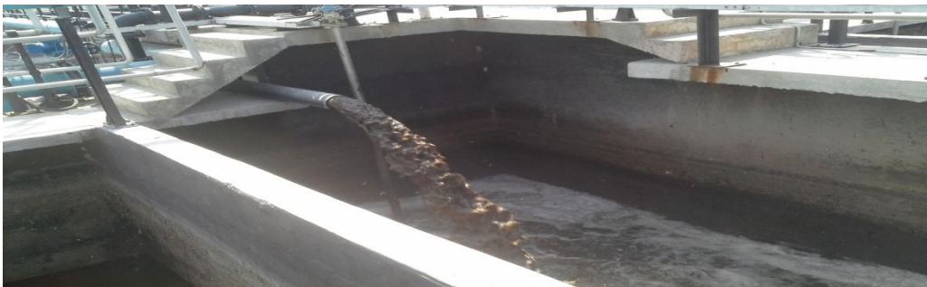
Fig 3.15 Reactivated Sludge Mixing
