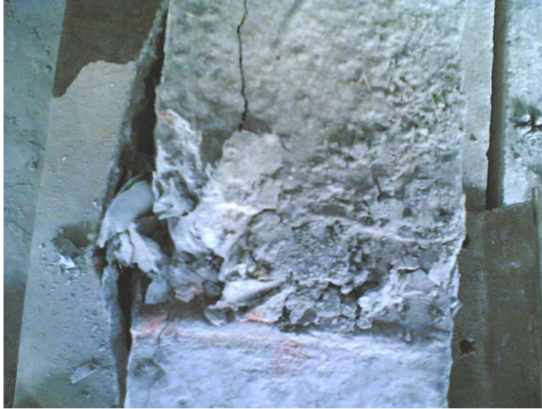
Plate 6.3 Crushing of Concrete in Balanced Beam Retrofitted with GFRP Jacketing
