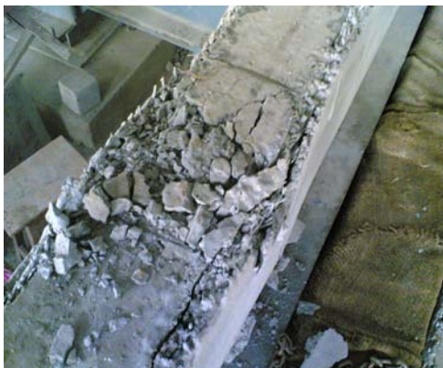
2B60(1)- Failure 2 (Crushing of Concrete)
