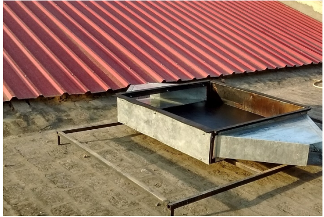
Fig 4.6: Absorber and Insulation installed in collector.
