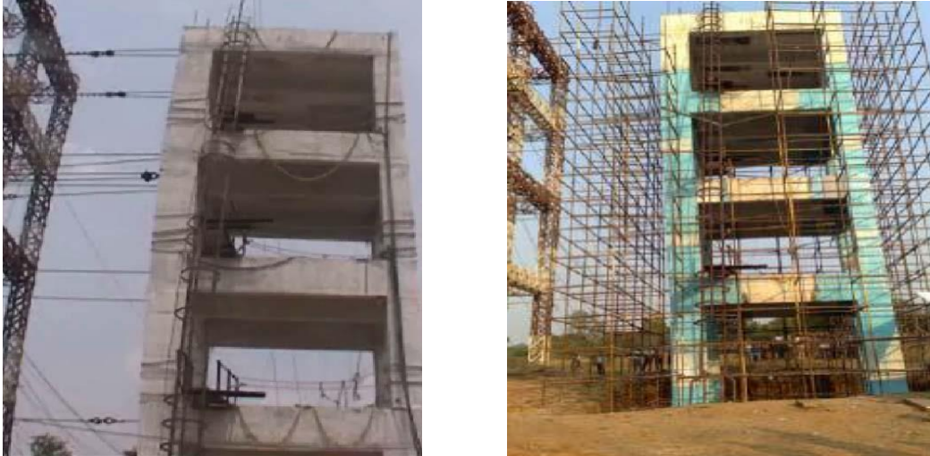
(a) (b) Figure 2.2: Full Scale Structure (a) As-built (b) Retrofitted Sharma et al. (2010)
