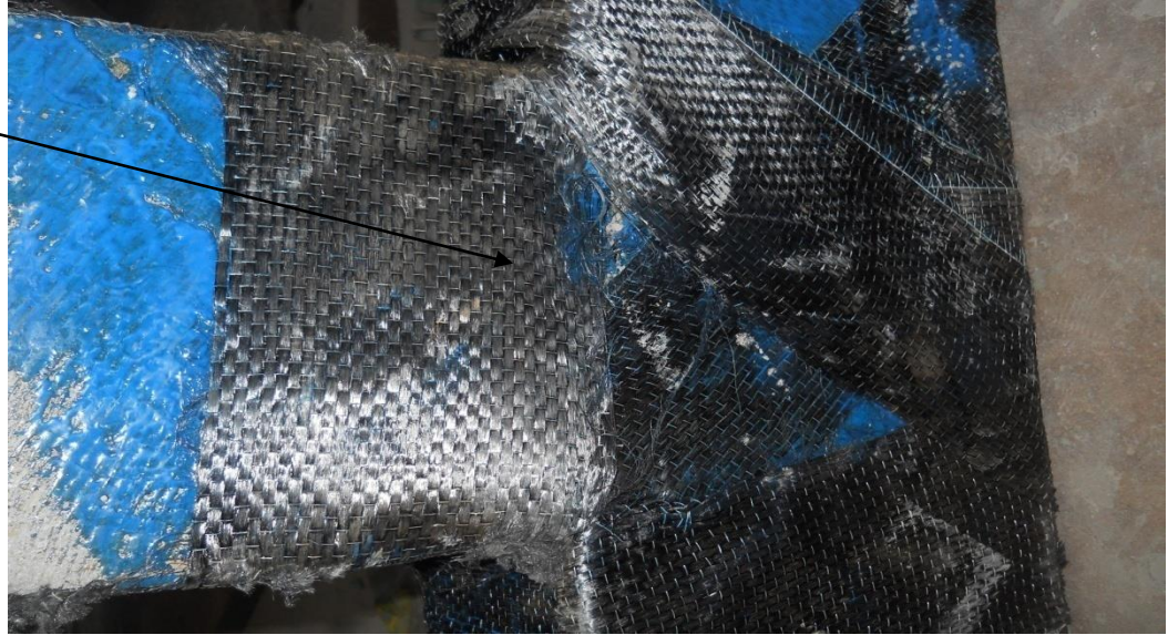
Plate 5.10: Failure of Beam-Column Joints without Debonding
