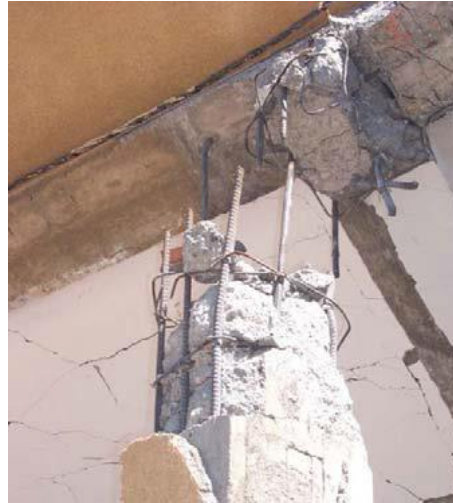
(b) Inadequate Reinforcement Anchorage
