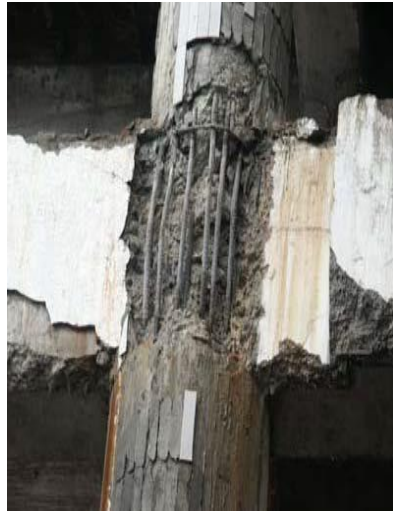
(a) Joint Shear Failure
