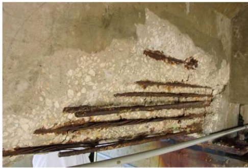
(a) Corrosion damage to a concrete beam
