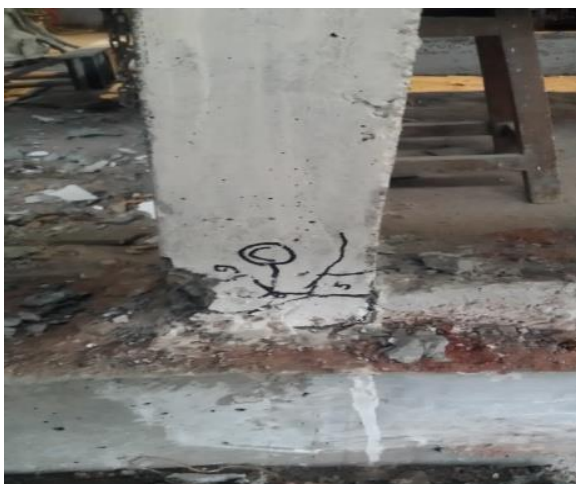
(g) Cracks in Column hinge C
