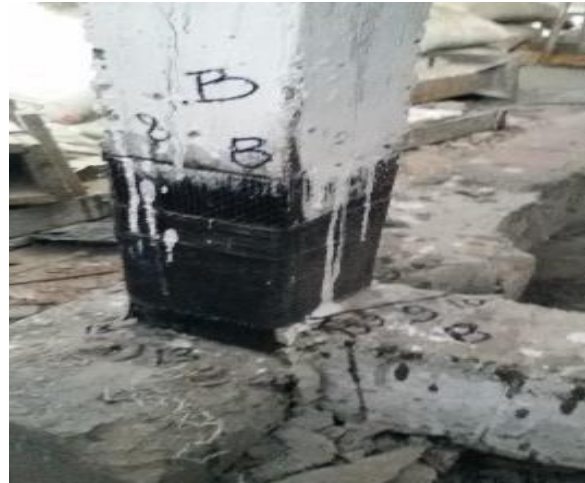
(b) Cracks in Column B
