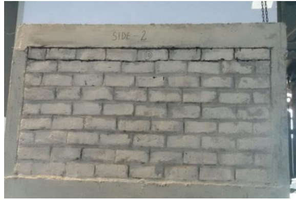
(i) Cracks in brick infill
