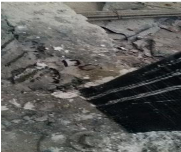
(c) Cracks in Column C
