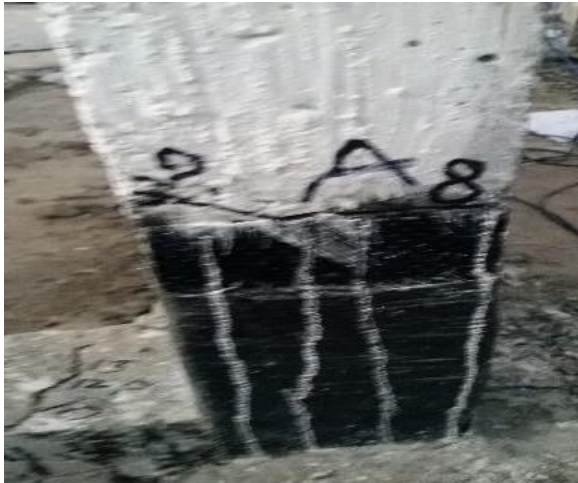
(a) Cracks in Column A
