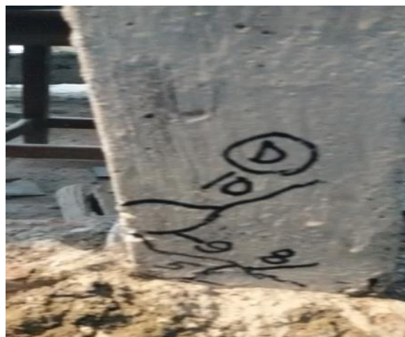
(h) Cracks in Column hinge D
