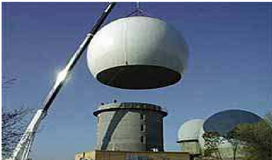
Fig.1.14(c) FRP radar dome (25m diameter, factory made FRP sandwich panels are bolted together on site) [21]
