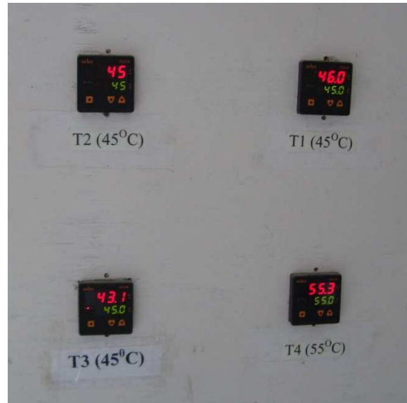
Fig. 4.8 Temperature display panel with controllers
