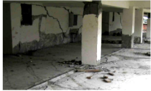
Fig-2.4(b) In-plane infill failure in yinxiu
