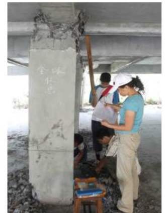
Fig-2.2(c) Typical column damage.
