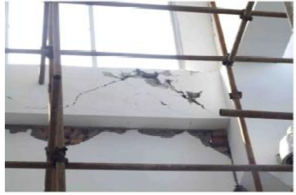
Fig-2.1(b) Beam failure due to overstressing
