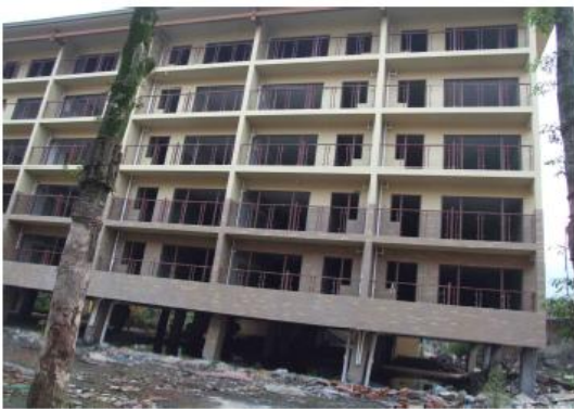
Fig-2.2(a) Leaned 6-story building in Duiiangvan
