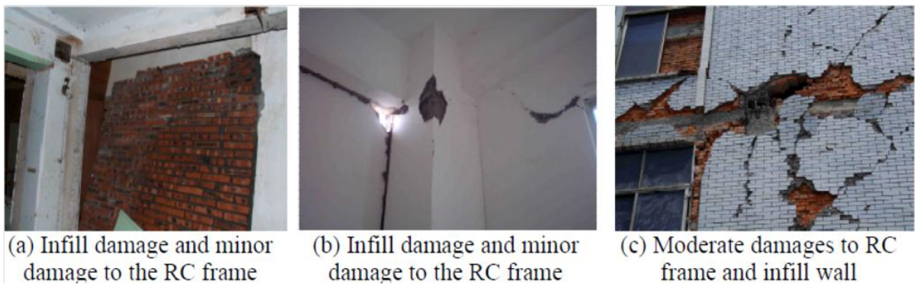
Fig-1.2, Effect of solid infill walls on the behavior of the bounding RC frame (Bixiong, Li et al. (2008))
