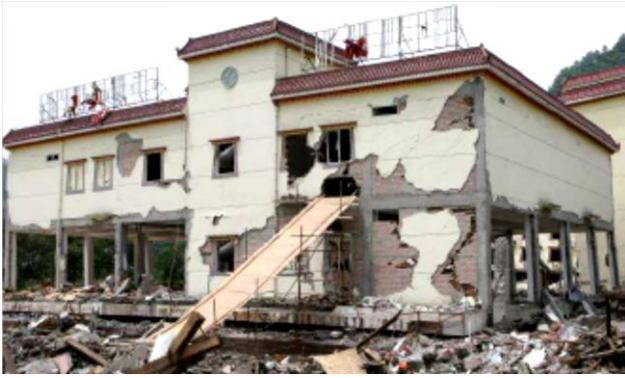
Fig-2.4(a) Partial collapse of 3-story RC frame building with masonry infill walls in Yingxiu
