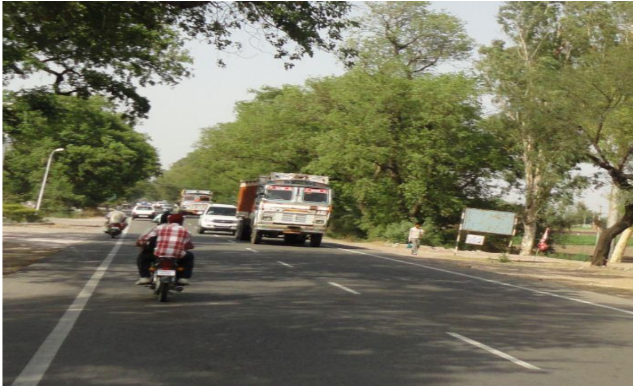
Inadequate Width of Highway Section
