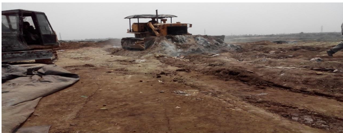
Figure 2.7: Waste disposal in secured landfill
