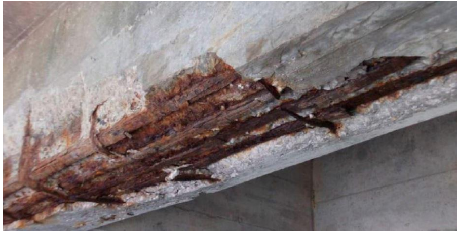
Figure 1. 1 Severely corroded reinforcement bars degrading the performance of RC structure (Duvnjak et al. 2021)
