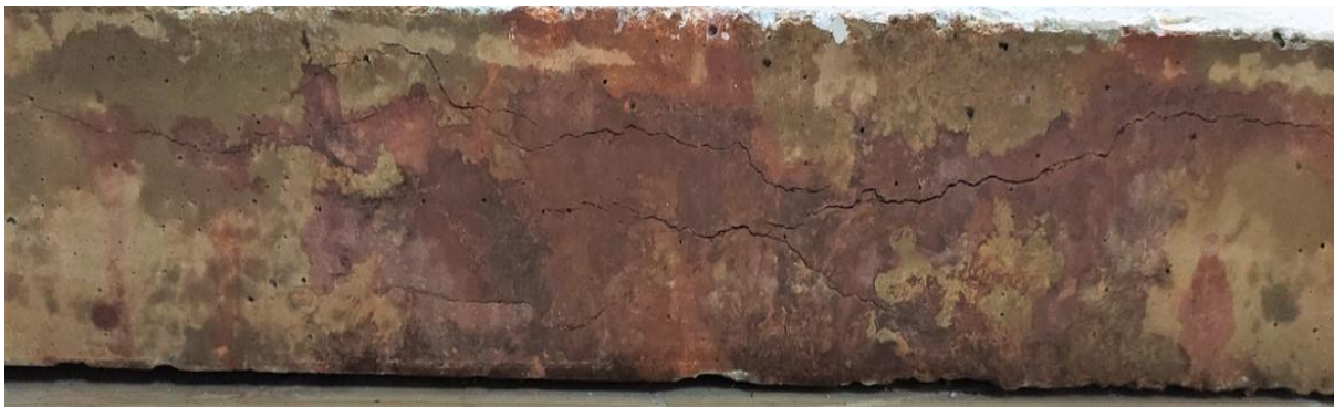
(i) Wider cracks along the longitudinal surface of the column
