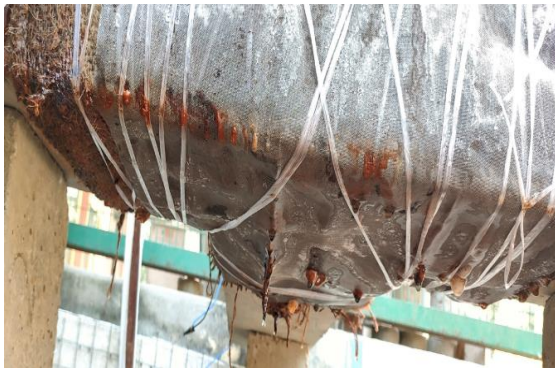
(a) Initial stage of corrosion
