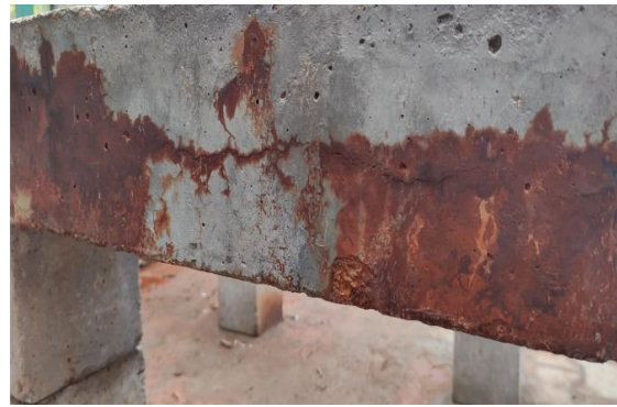
(b) Hairline cracks due to corrosion
