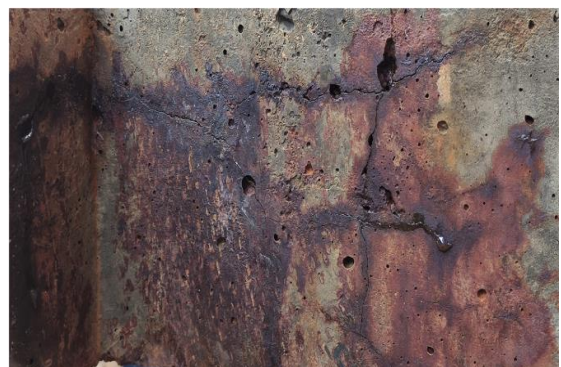
(f) Wide cracks at higher levels of corrosion
