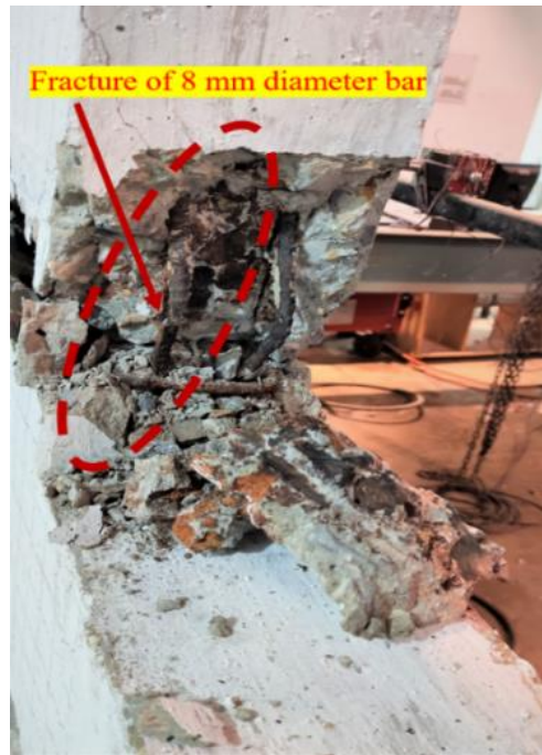
Figure 4. 11 Fracture of corroded reinforcement bar
