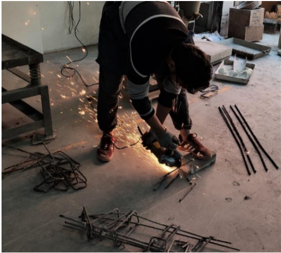
(a) Corroded bars of desired length were cut
