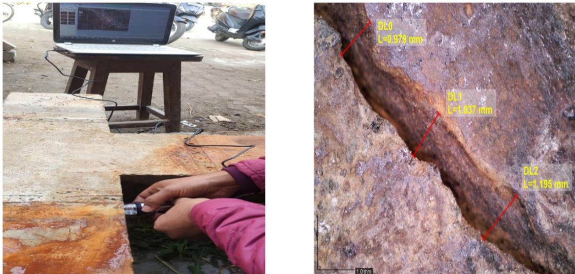
Figure 3. 8 Crack monitoring and measuring via Dino-Lite edge digital microscope
