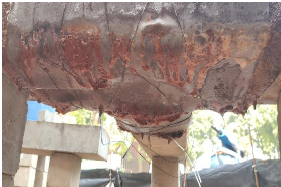
(c) More rust deposition
