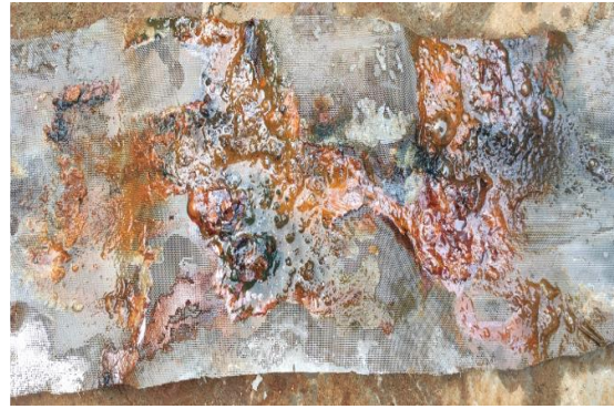
(h) Deposited rust on the mesh surface
