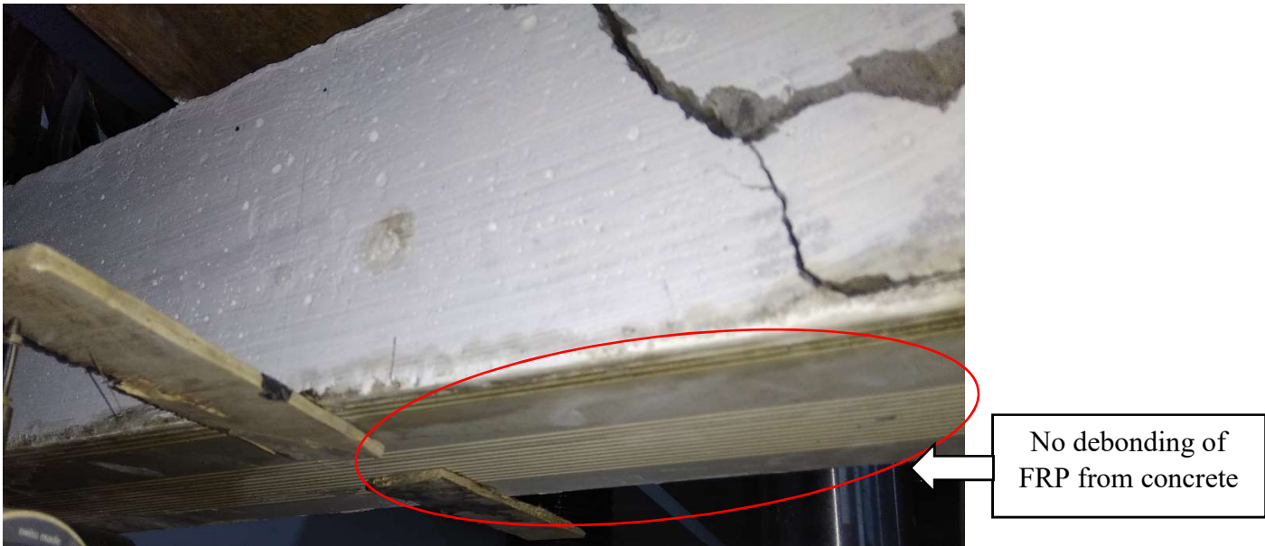
Fig 4.5 Condition of joint at failure in specimen BC
