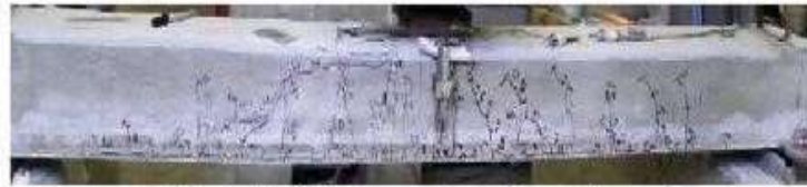
2) Hybrid failure mode of specimen 5
