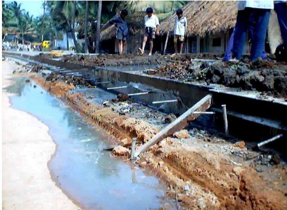
Fig1.3b Tie roads are used for longitudinal (D.V .Bhavanna Rao)
