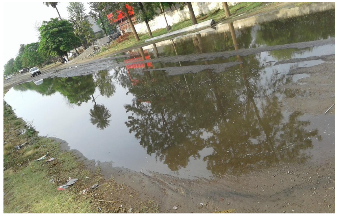
Fig. 3.6: Water on carriageway of Road Section UR04
