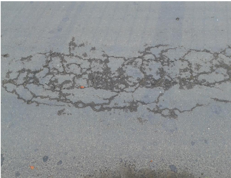
Fig. 3.16: Cracks on Section UR04
