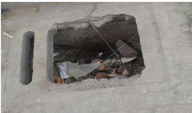
Fig. 3.4: Choked Drain on Road Section UR01
