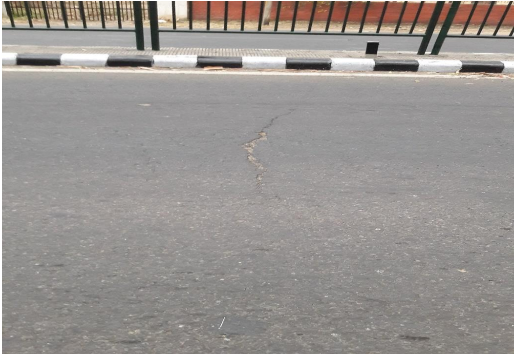
Fig. 3.14: Transverse Cracking on Road Section
