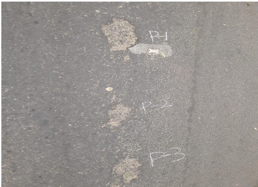
Fig. 3.20: Pothole on Section UR04
