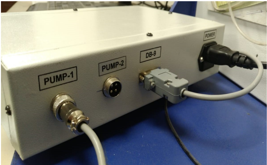
Fig 3.4 various connection on pump controller
