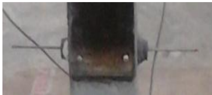
Figure 3.10: Insulators used for safety purpose
