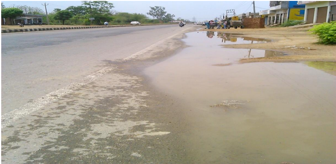
Fig.7.1: Poor drainage condition at Chainage 91(No longitudinal drain)
