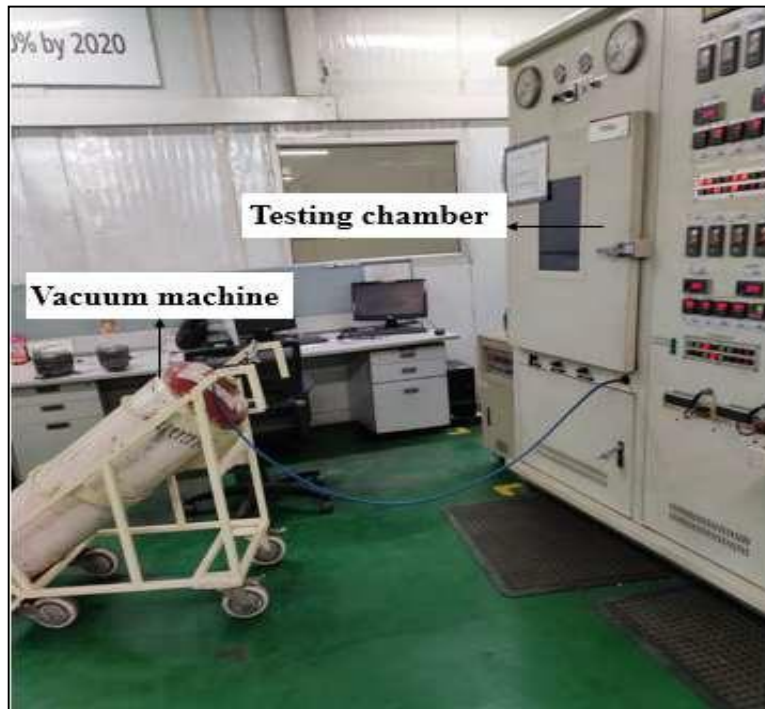
Fig. 20: Vacuum process of Compressor [LG. Electronics, India]
