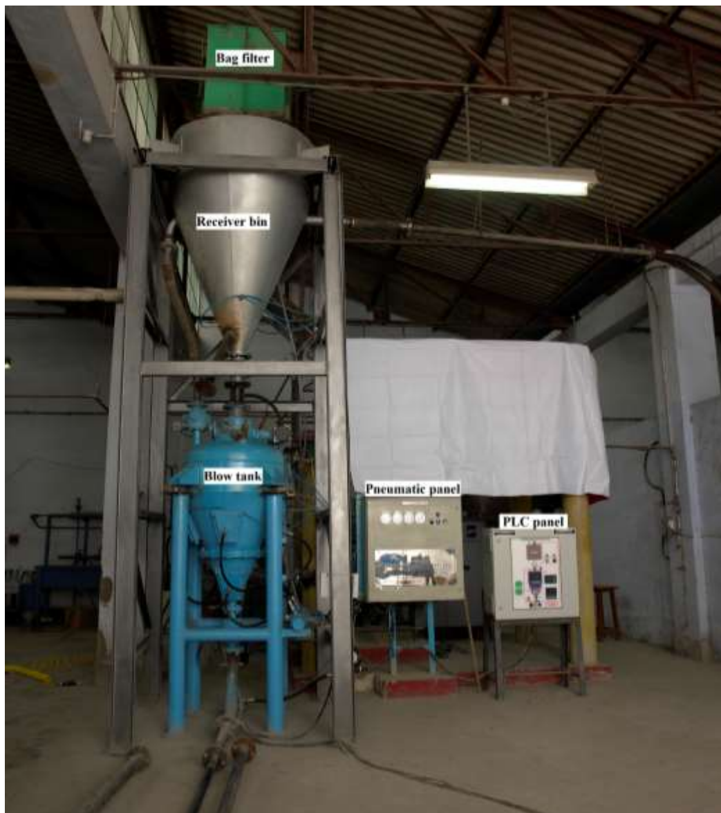
Figure 2.2: Blow tank, receiver bin, bag filter, pneumatic panel, and programmable logic controller (PLC) panel
