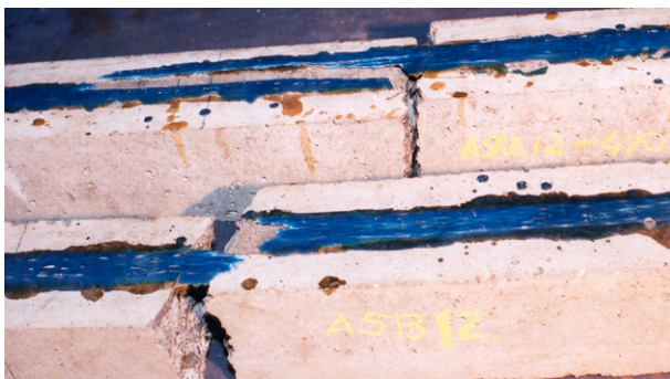
Fig. 10. Debonding and rupture of sheet for pre-cracked beams conditioned outdoors (ASB12-350 and ASB12-470).
