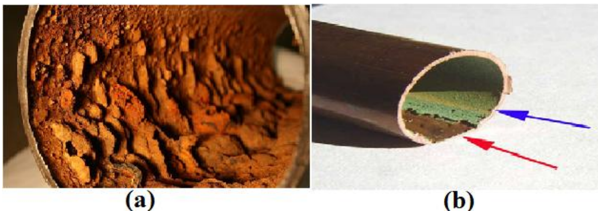
Fig 1.3 (a) MIC corrosion inside a fire sprinkler systems.
