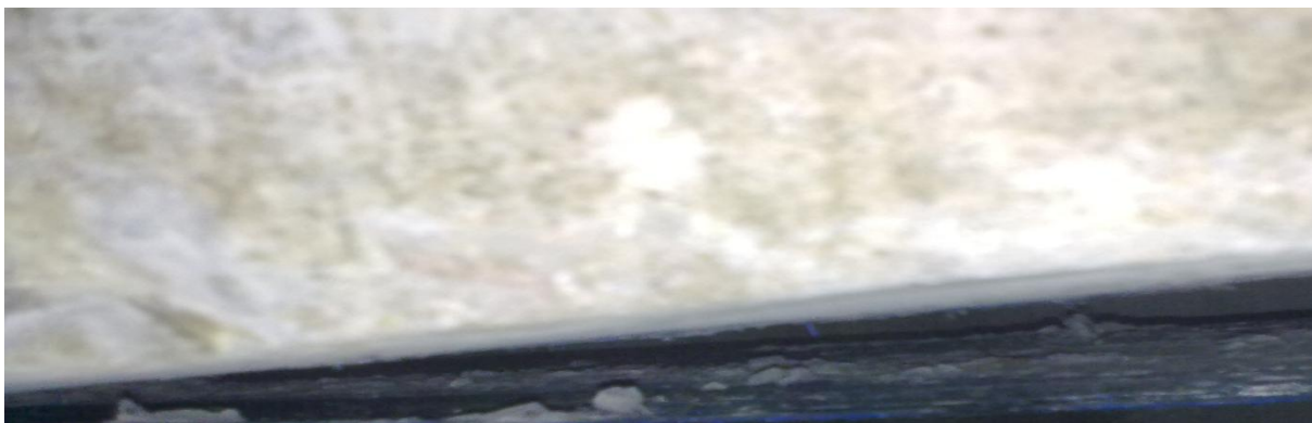
Fig 4.16: Failure of DB12 by debonding of sheets
