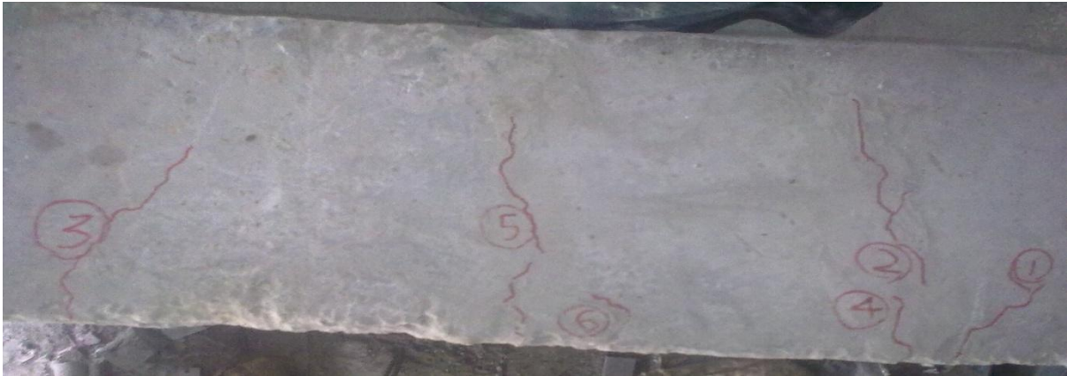
Fig 4.4: Crack pattern observed after CB02 is failed
