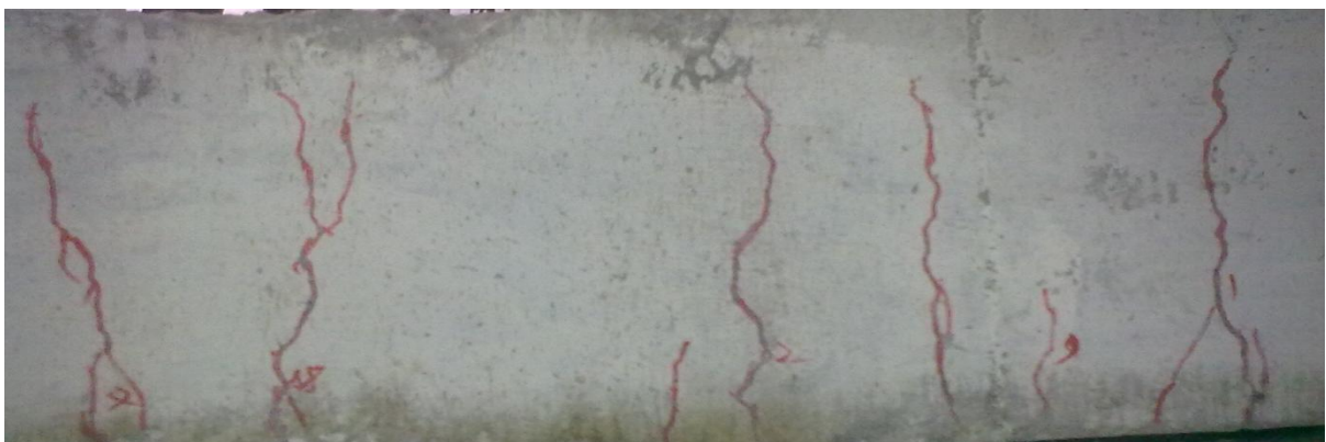
Fig 4.17: Cracking pattern of DB12
