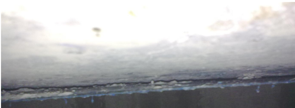
Fig 4.20: Failure of DB31 by debonding of sheets
