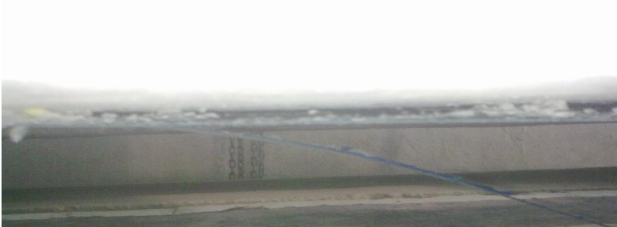
Fig 4.13: Failure of DB12 by debonding of sheets
