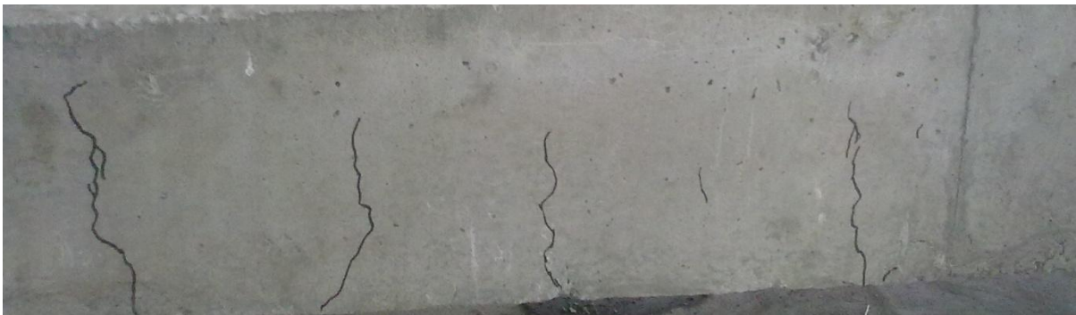
Fig 4.2: Crack pattern observed after CB01 is failed
