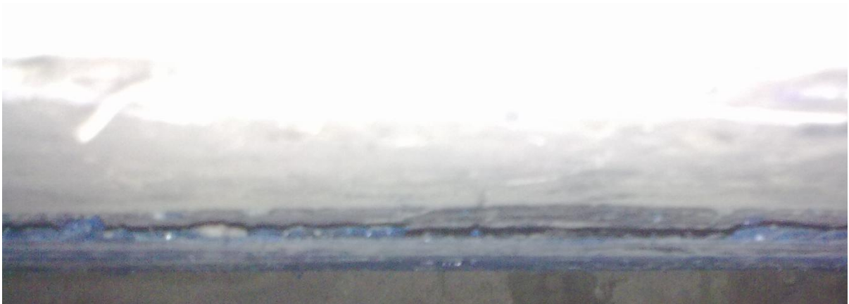
Fig 4.23: Failure of DB32 by debonding of sheets
