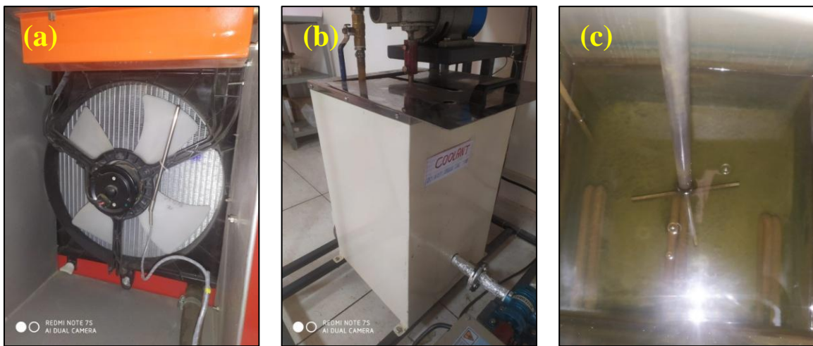
Figure 5: (a) Radiator and Fan assembly, (b) Storage tank, (c) inside view of the tank showing heating elements and stirrer
