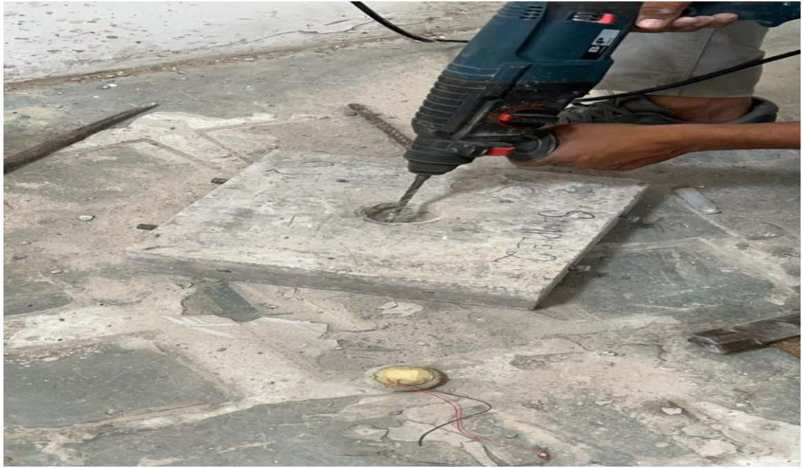
Figure 3. 12 Drilled a hole to place anode at the center to the level of steel
