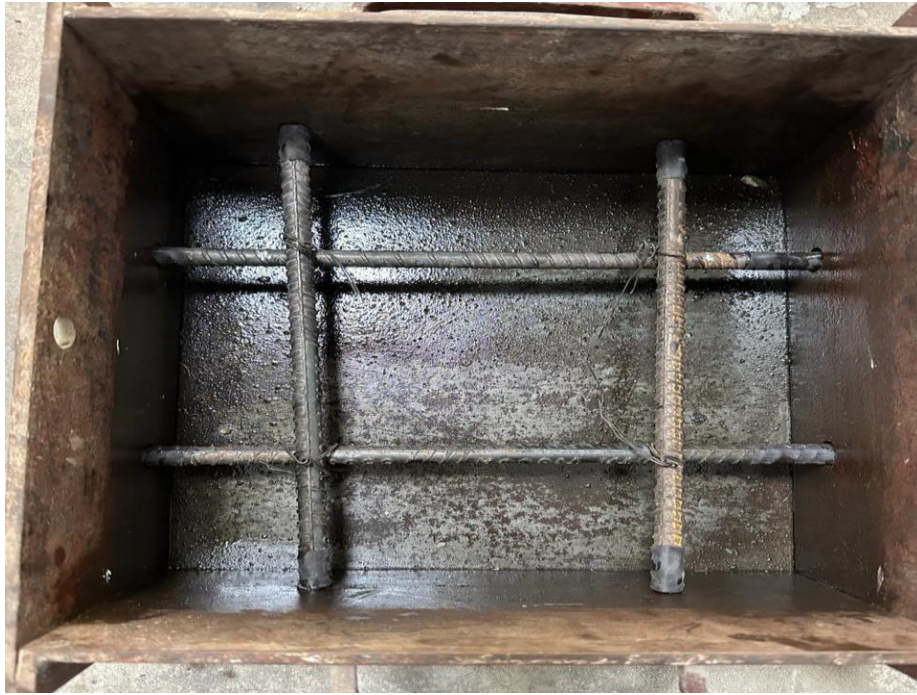
Figure 3. 10 4 Steel bar of 12mm were placed and are connected through tie wire
