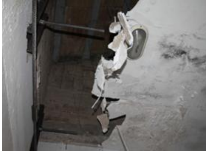
Figure 2.13: Damage to plasterboard ceiling system [10]
