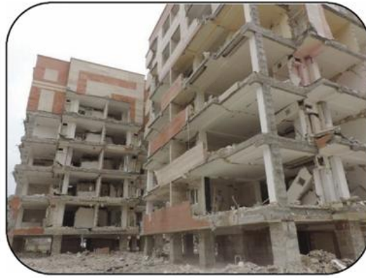
Figure 2.8: Extensive damage to non-structural components during earthquake [5]
