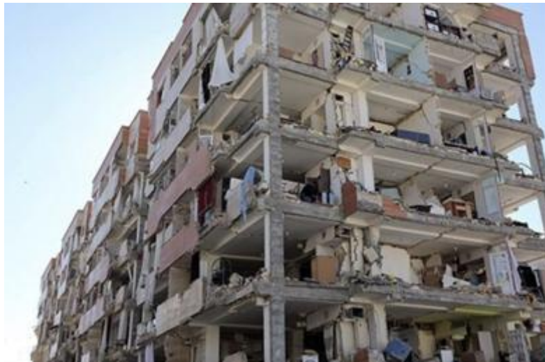
Figure 2.5: Extensive damages to exterior and facade walls of buildings despite the acceptable performance of the lateral load-bearing systems in the Kermanshah earthquake, 2017 [3]
