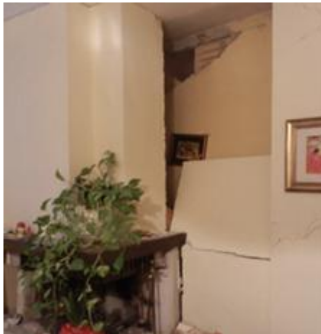
Figure 2.12: Typical damage to masonry infills. internal partition [10]
