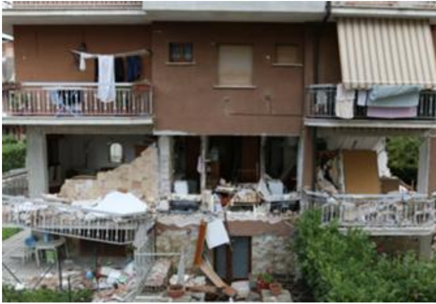
Figure 2.11: Collapse of infill panels [10]
