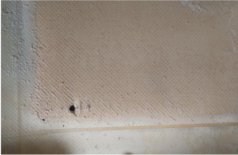
Figure 6.3: Perforation on membrane sheet
