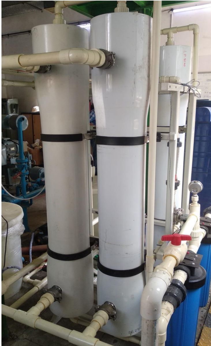
Figure 5.2: Initial setup of Ultrafiltration unit
