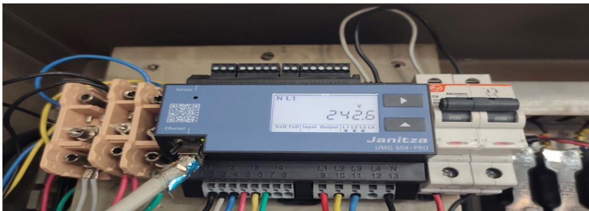
Fig.1.2 ZED/ Power analyser installed at the DG area at a Transformer bus
