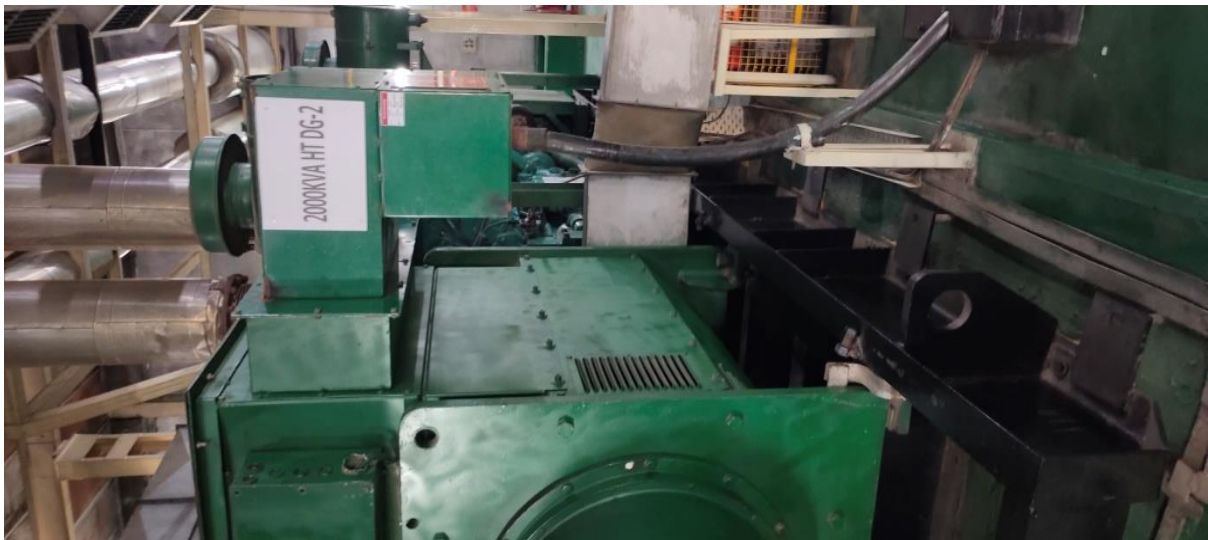
Fig. 4.6 Image of 2000KVA HTDG installed at the electrical facility of LG plant of Noida
