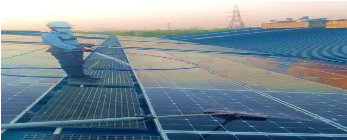
Fig. 4.2 Solar module cleaning at the LG plant, Noida
