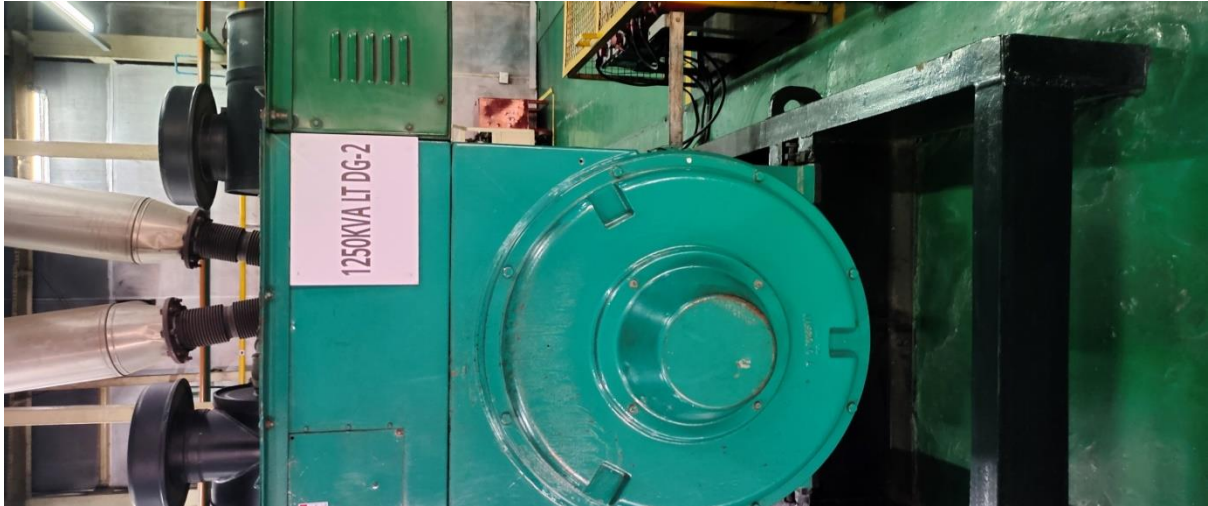
Fig. 4.5 Image of 1250KVA LTDG installed at the electrical facility of LG plant of Noida
