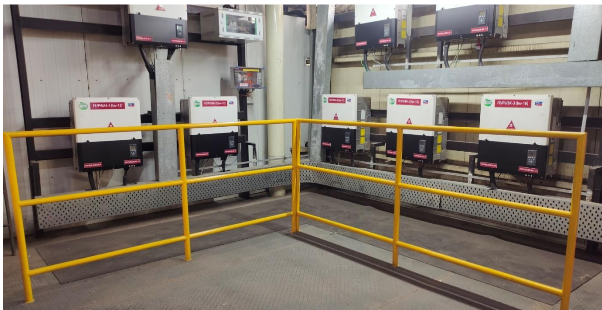
Fig. 2.6 various solar inverters installed at the Bulk store of LG plant
