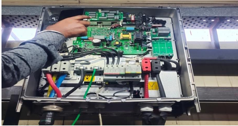
Fig. 2.3 Solar Inverter some fault detection
