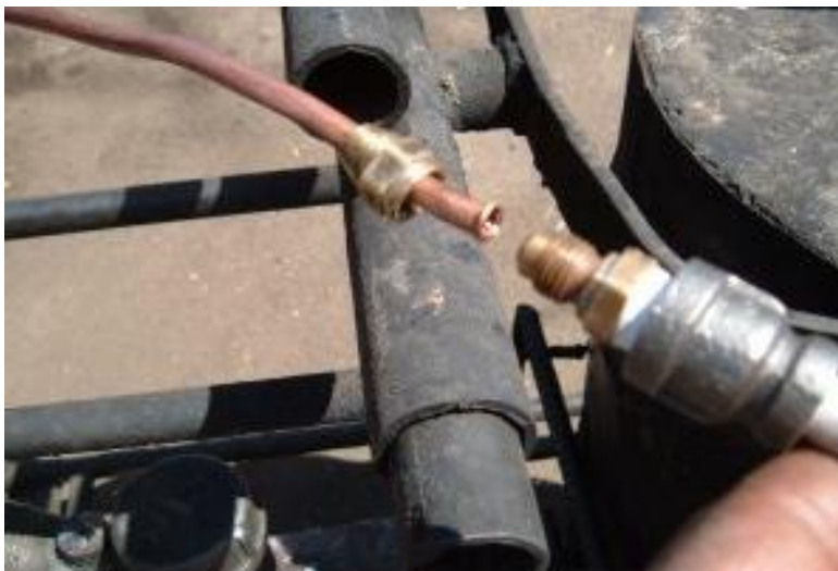
Figure 5.19: Flared connections tubes and nuts in system [RAC Lab, Thapar Uni.]
